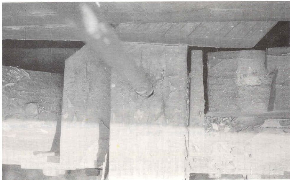
“Shrinkage in the bottom chord connected with wedges.”
