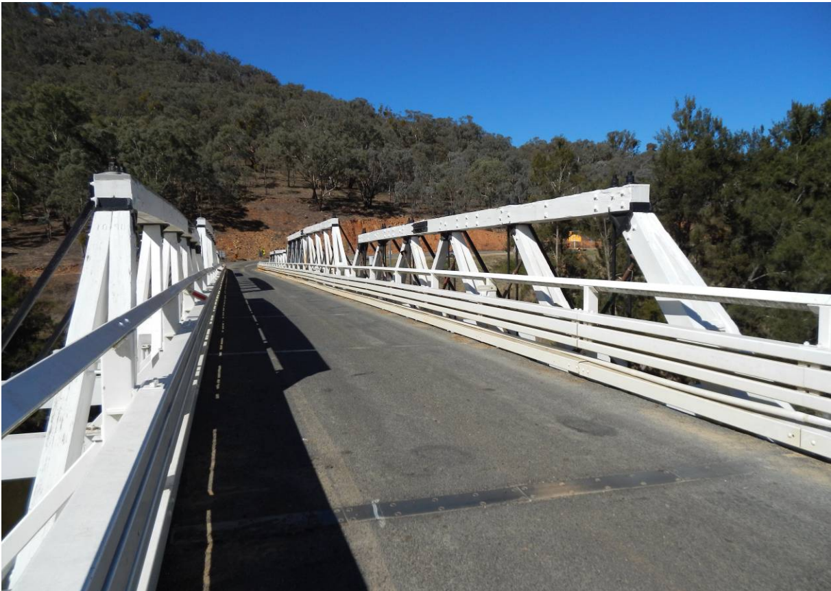
Figure 154: Barriers of same style as above, but more attention drawn from truss due to colour
