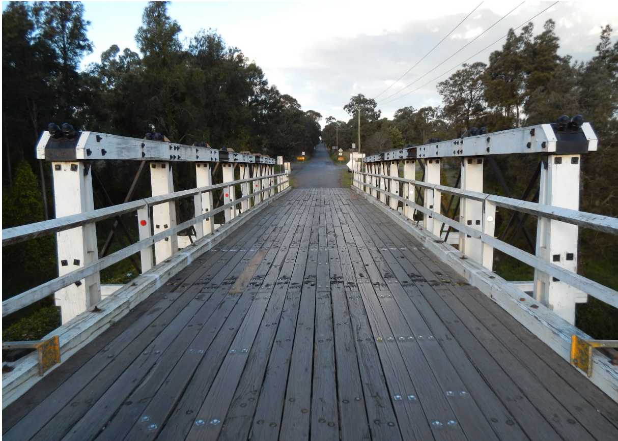
Figure 49: Gillies Bridge - Short Span Council de Burgh truss over Black Creek near Cessnock
