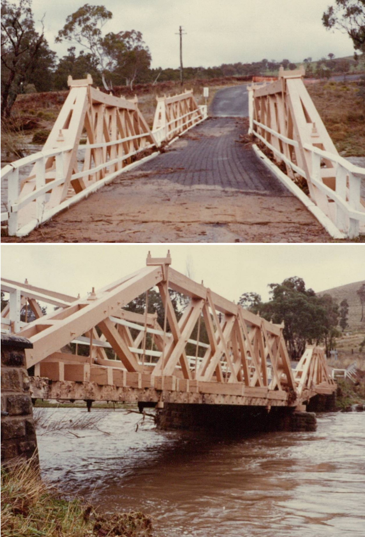
Figure 186: Flood Damage to Central Pier of McKanes Bridge over the Cox’s River near Lithgow
