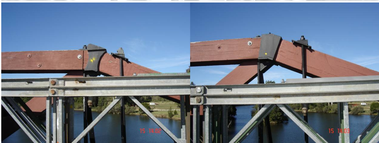
Figure 180: Top: Shoe Broken in 1975; Left: Original Shoe Remaining; Right: Steel Shoe Installed 1975
