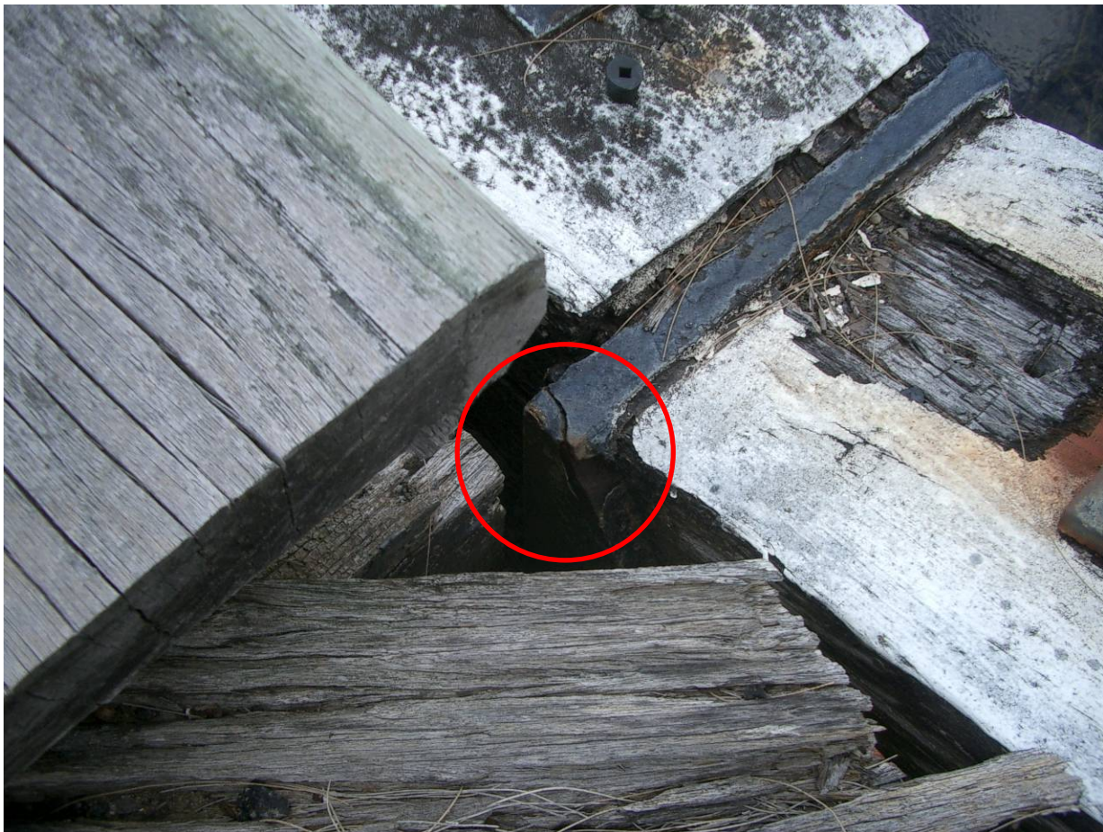
Figure 108: Fractured Cast Iron Shoe at Base of Principal on Monkerai Bridge (2012)
