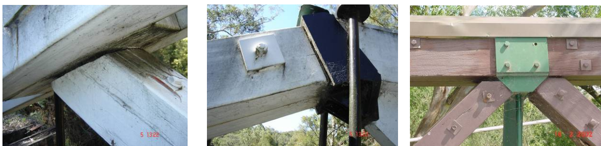
Figure 123: Gaps opening up in McDonald Truss Connections (Galston and Junction Bridges)
