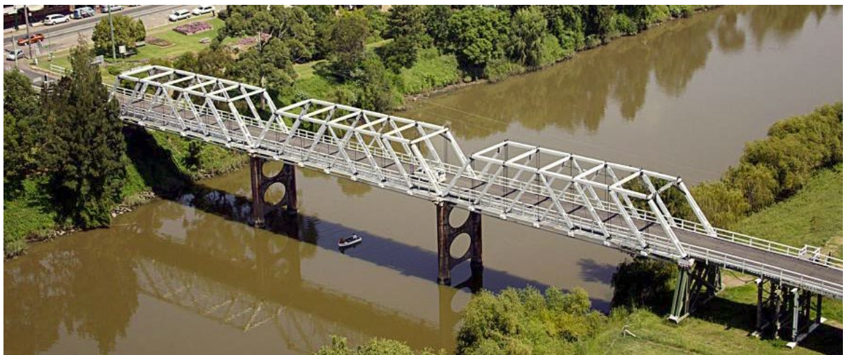
Figure 41: Allan Truss: Morpeth Bridge over the Hunter River near Maitland with Overhead Bracing
