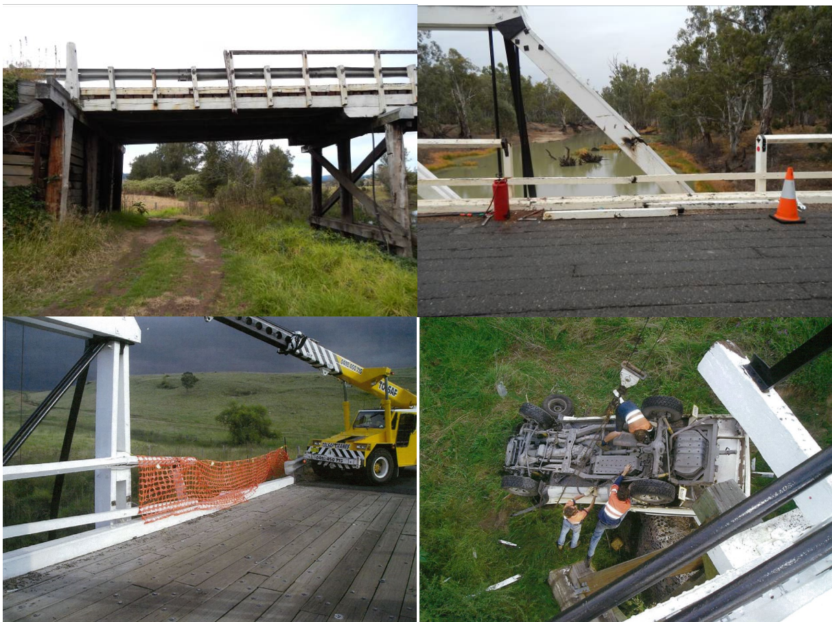
Figure 150: Typical Failure of Timber Barriers Under Impact Loading
