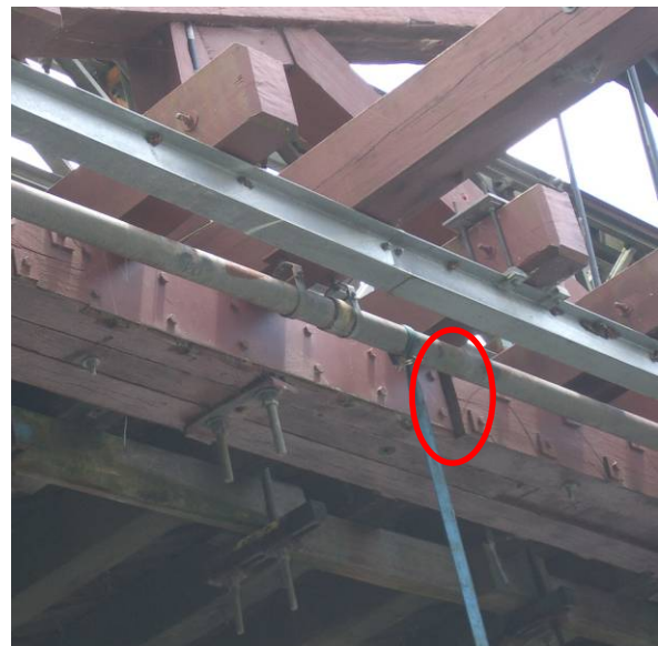
Figure 70: Clarence Town Bridge (Old PWD) – bottom chord notched on side to fit splice plate
