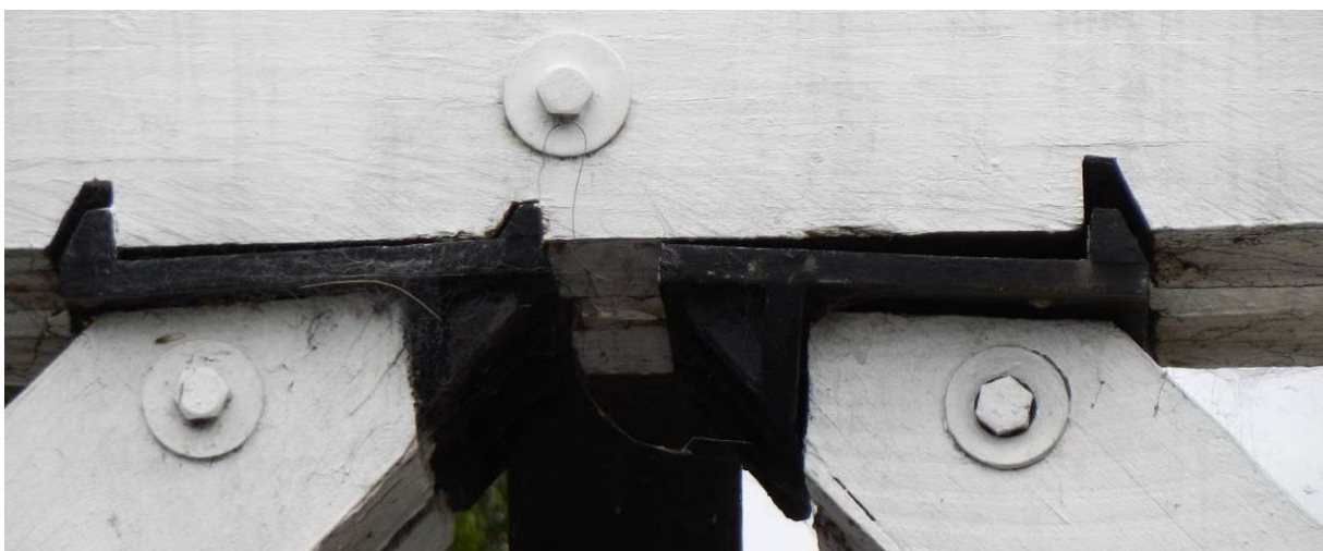
Figure 146: Separation of Shoes from Top Chord in Dare Truss over Williams River, Cooreei Bridge
