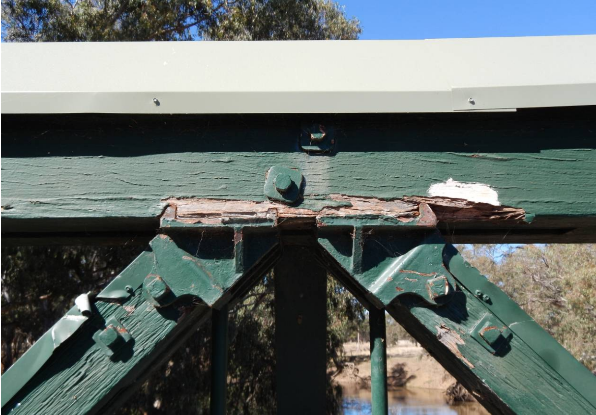
Figure 144: Deterioration at Top Chord Shoe in Dare Truss at Warroo
