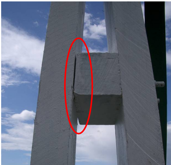
Figure 69: Tabulam Bridge (de Burgh) – difficulty fitting spacer due to cup of left-hand timber flitch
