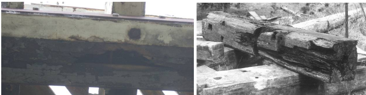
Figure 95: Left: Monkerai Bridge Bottom Chord; Right: Clarence Town Bridge Butting Block
