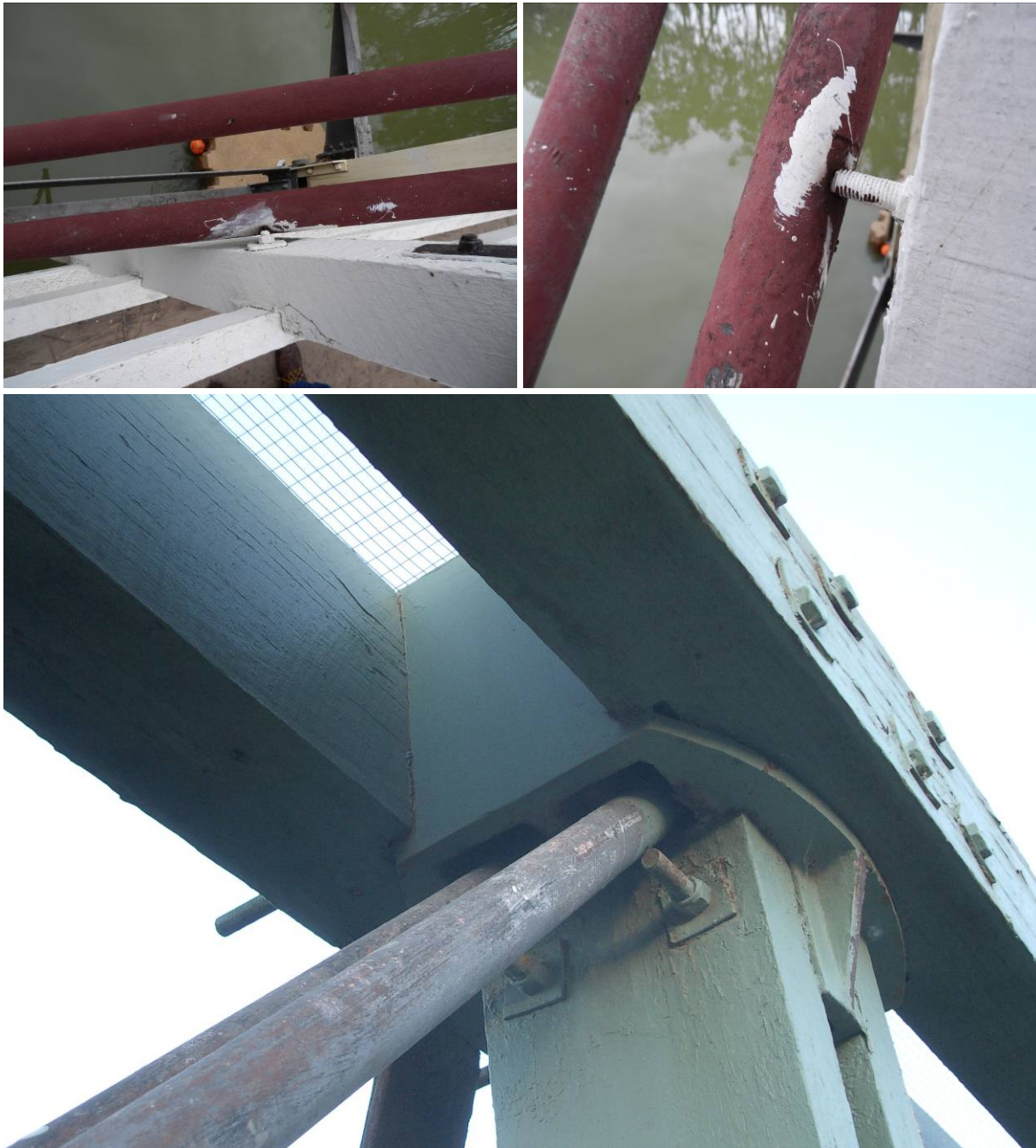
Figure 142: Damage to de Burgh Truss Tension Rods due to Nearby Bolts and Vibration Effects.
