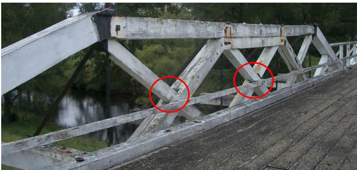
Figure 109: Oversize notched joints on Monkerai Bridge to allow Tightening and Recambering
