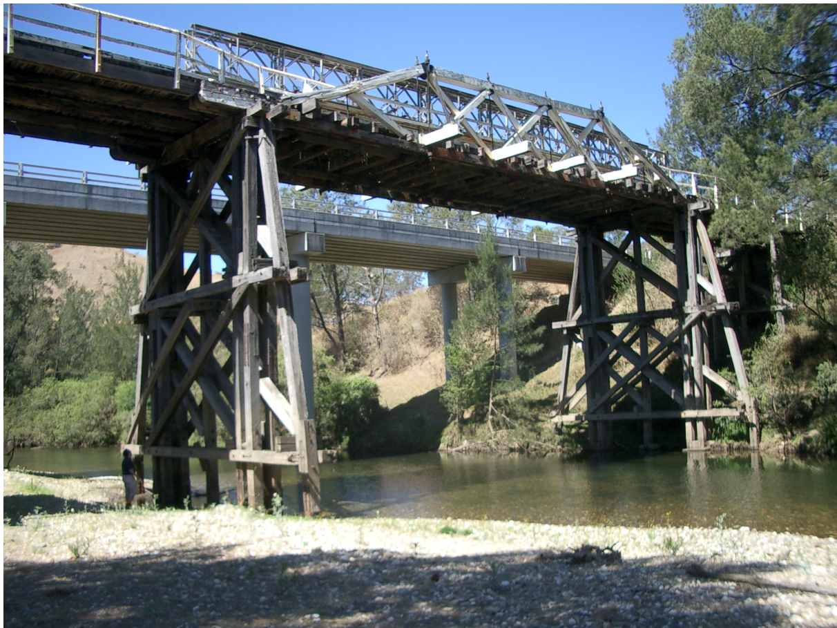
Figure 33: McDonald Truss over Five Day Creek with new Concrete Bridge in Background
