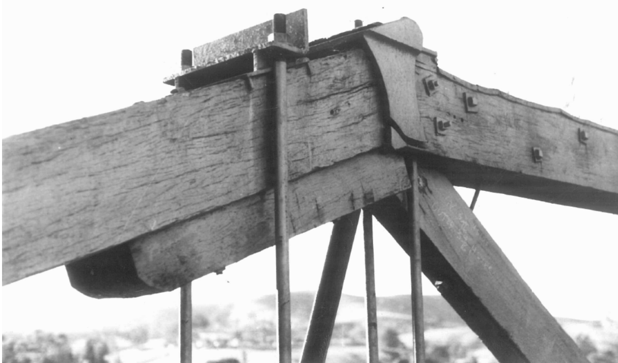
Figure 93: Clarence Town Bridge – Fractured Cast Iron Shoe and Supplementary Tension Rods
