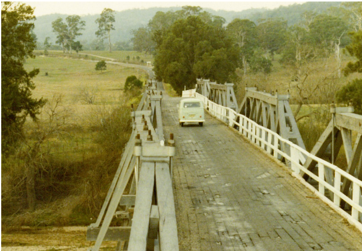
Figure 114: Loss of Lateral Stability in sagging McDonald Truss over Bega River at Tarraganda
