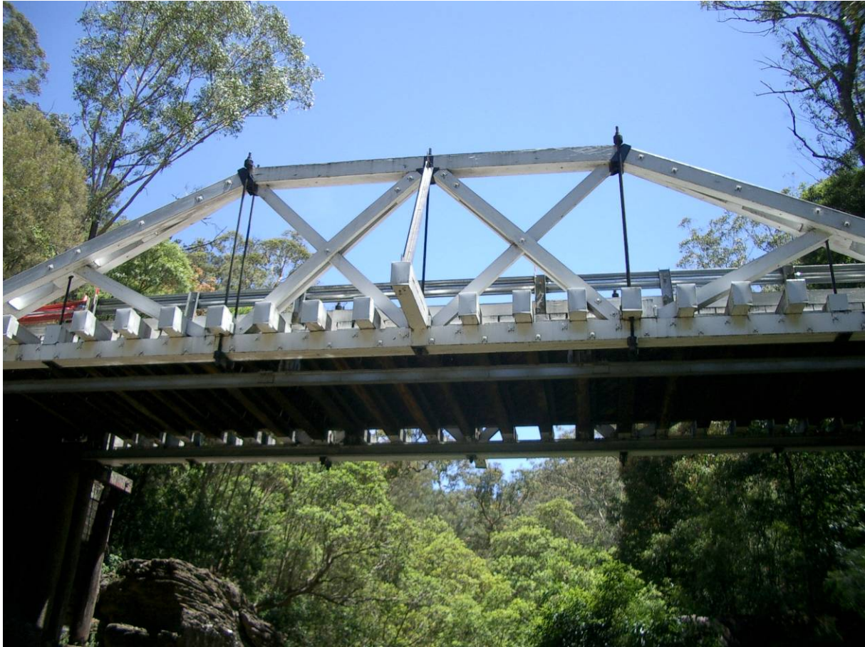
Figure 195: External Steel Plates used to Strengthen Bottom Chord of Galston Gorge Bridge
