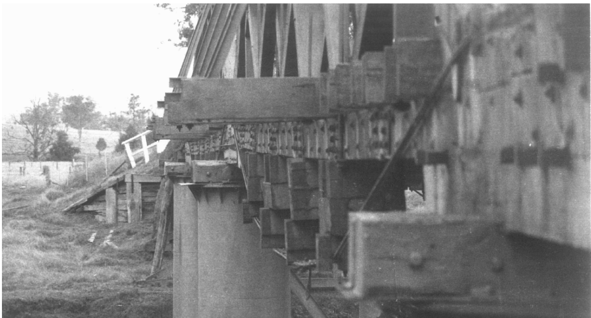
Figure 94: Clarence Town Bridge – Sagging of Bottom Chord with Supplementary Under-Trussing
