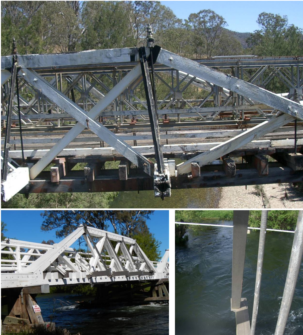
Figure 190: Additional Sway Bracing (top) Five Day Creek, (bottom) Junction Bridge Tumut River
