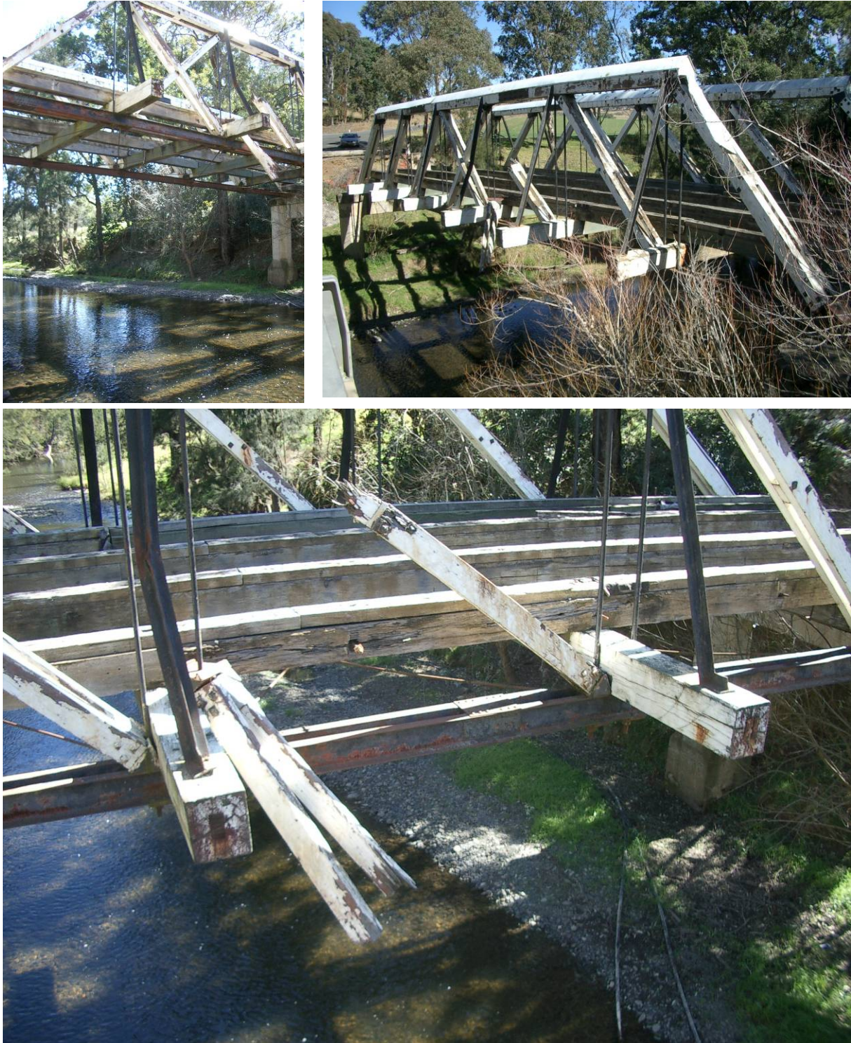
Figure 128: Impact Damaged Dare Truss near Moonan Flat
