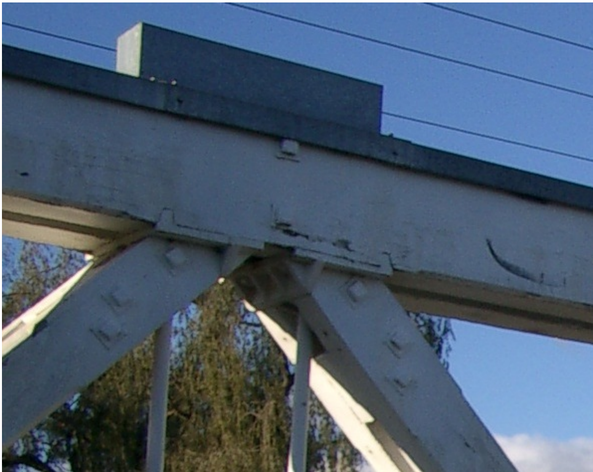
Figure 143: Deterioration at Top Chord Shoe in Dare Truss at Bendemeer
