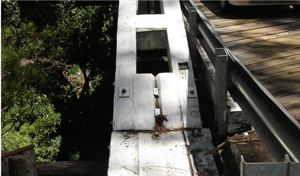
Figure 118: Large Spacer replaced with Two Laminates and Shear Keys at Galston – Moisture Trap
