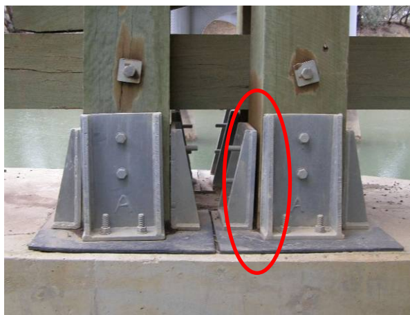
Figure 72: Carrathool Bridge (substructure) showing gap in connection due to shrinkage
