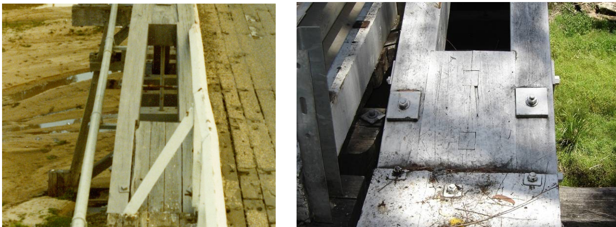
Figure 117: Three Laminates used for Spacer at Tarraganda, Two Laminates with shear keys at Galston
