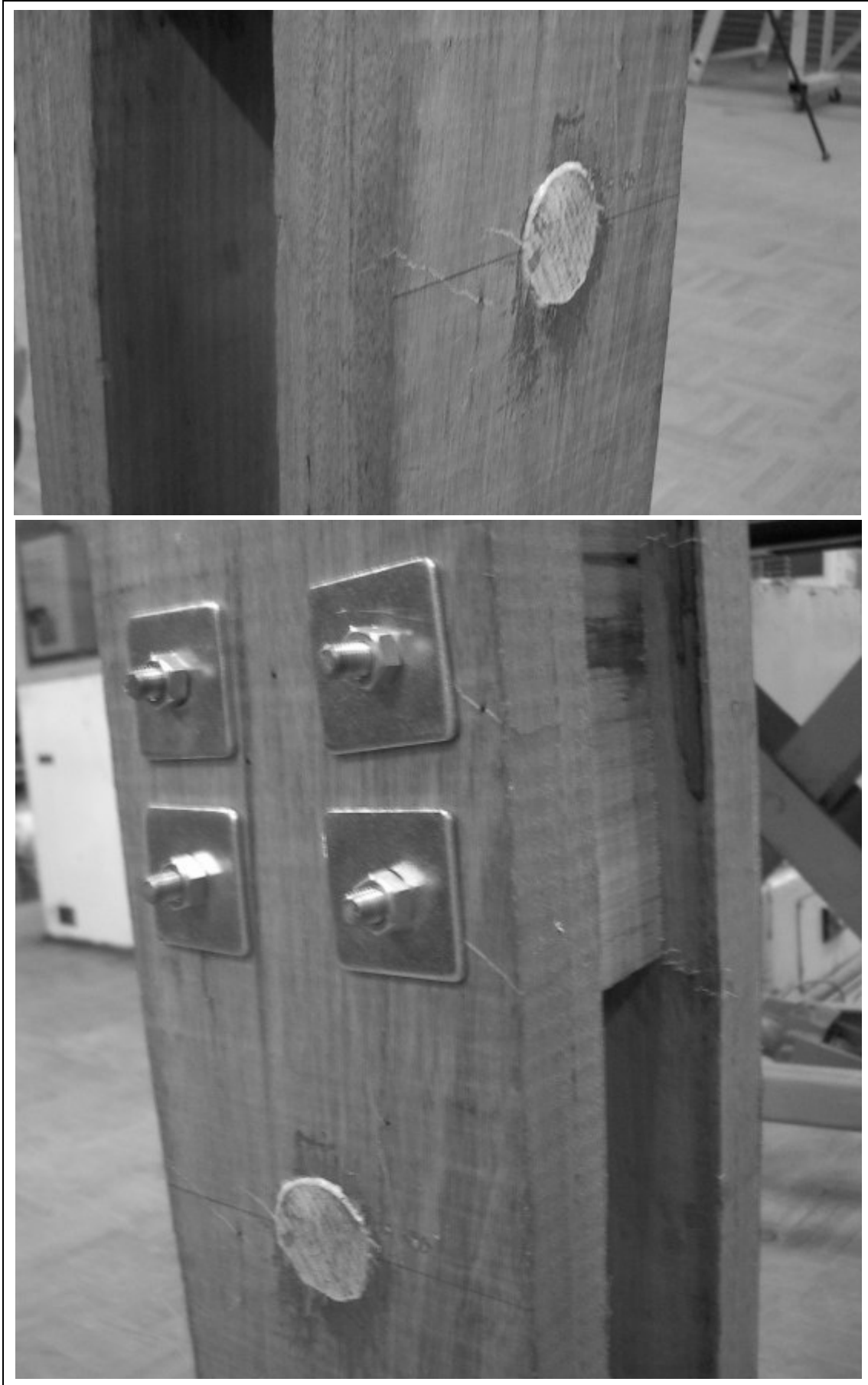
Figure A.9: Photographs of failure locations for Assembly 08A02A
