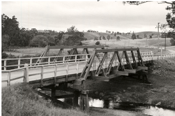
Fig 8. Nunnock Creek Bridge, near Bega, NSW (built 1897) detailing duplicate principals and diagonals (RTA Photo Archive).
