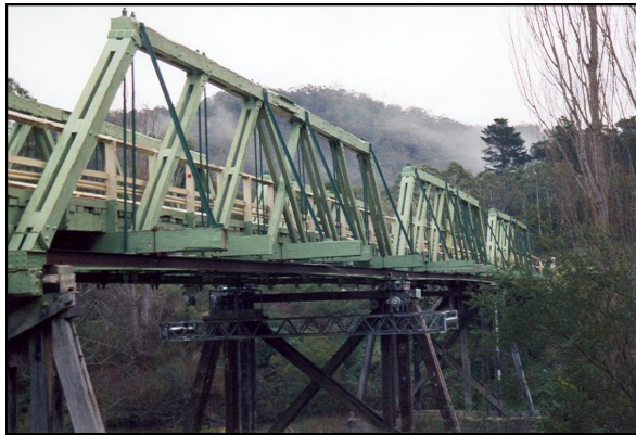
Fig 10. New Buildings Bridge over the Towamba River, near Wyndham, NSW (built 1921) has the characteristic steel bottom chord of a Dare composite truss (Author's collection). Note the principals and diagonals are no longer splayed as in the Allan truss.
