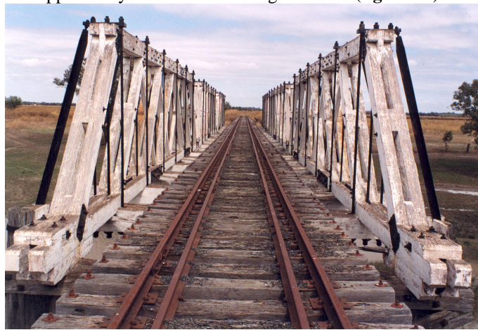
Fig 11. View of Two Mile Creek Bridge at Walgett, NSW (built 1908) photo courtesy of Don Fraser. Note the principals and diagonals (now parallel) are duplicated for ease of maintenance.
