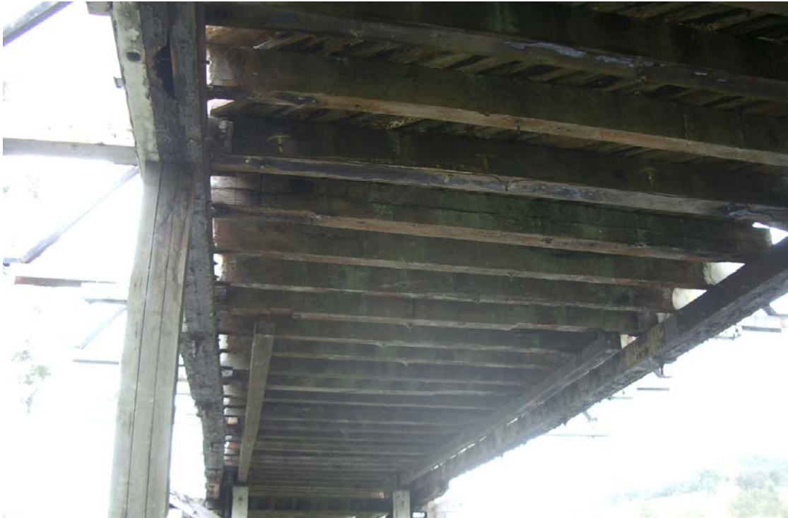
Figure 3-7: Photo showing poor condition and alignment of bottom chord.
