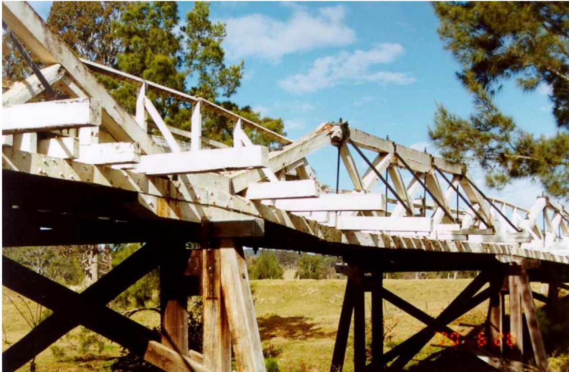
Figure 2-44: Failure of Principal and Bottom Chord in June 2000.
