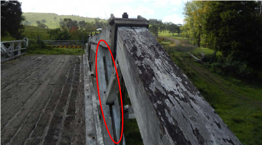
Figure 3-10: Photo showing gap and spacer introduced in double diagonal.
