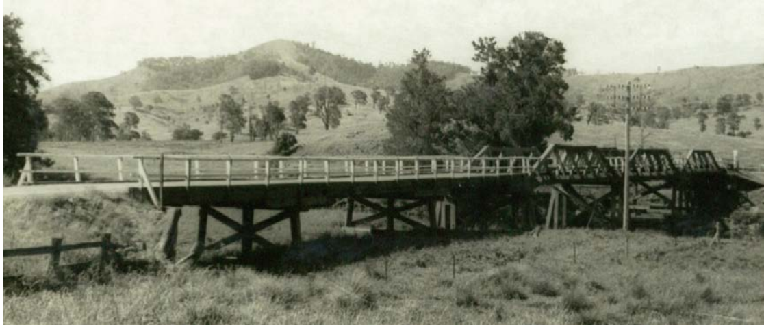
Figure 2-41: Before elimination of truss sags in 1967.
