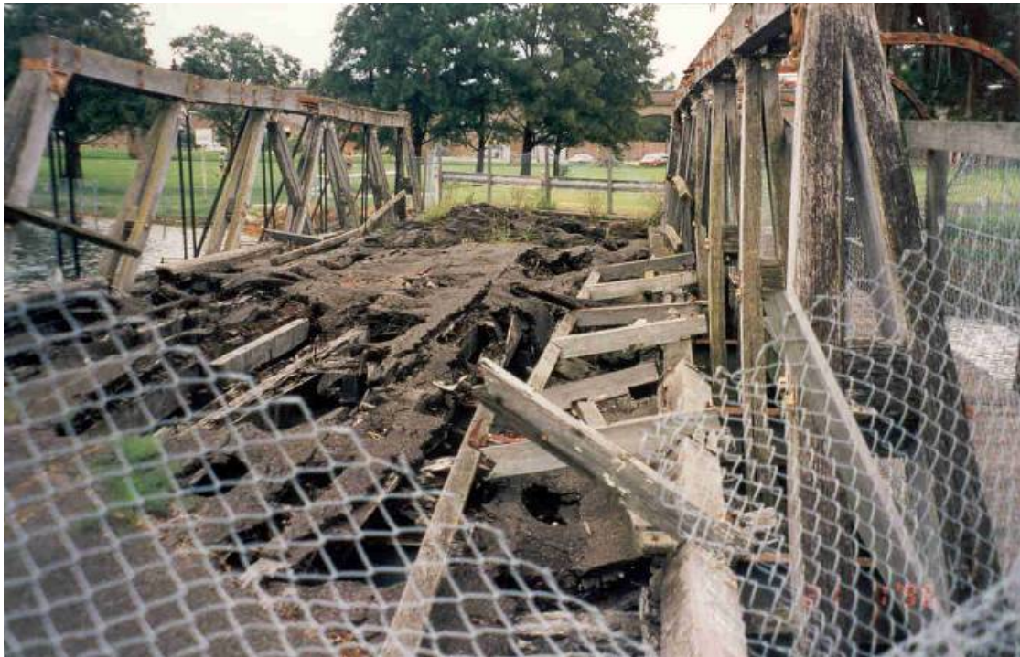
Figure 5-2: Johnston’s Creek Bridge, failed pedestrian bridge at Glebe.
