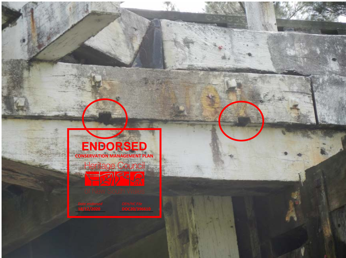
Figure 3-6: Photo of notches for missing shear keys in bottom chord.
