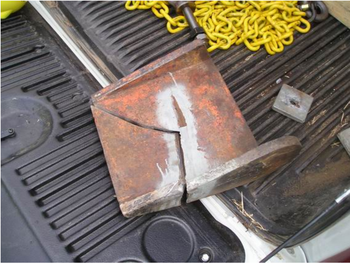
Figure 3-18: Photo of broken modified shoe removed from bridge.
