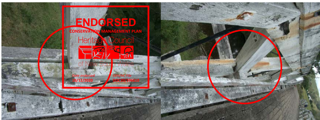
Figure 3-9: Photo showing oversize notches in timber diagonals.
