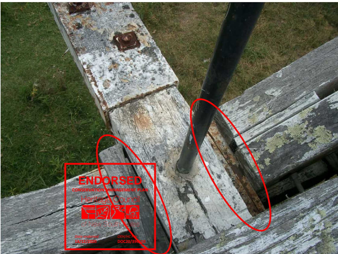
Figure 3-13: Photo of additional timber & metal wedges at base of diagonal.
