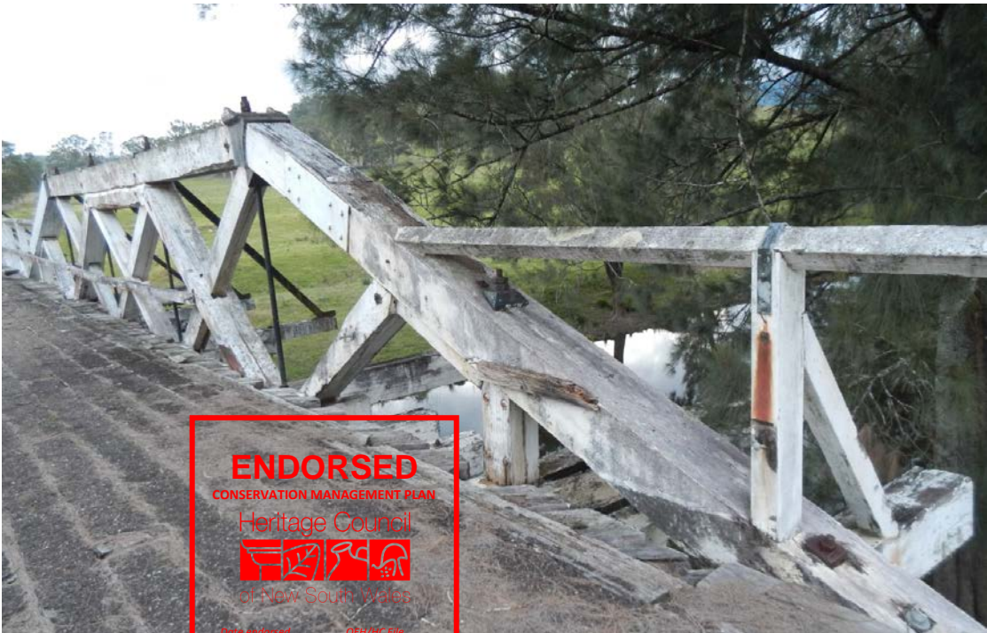
Figure 3-45: Photograph showing missing railings on truss span.
