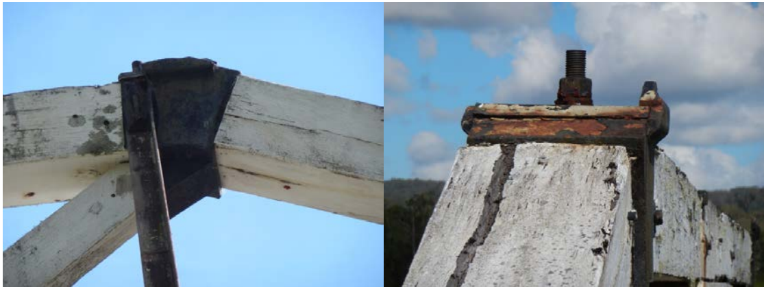
Figure 3-16: Photos of broken top chord cast iron shoes.
