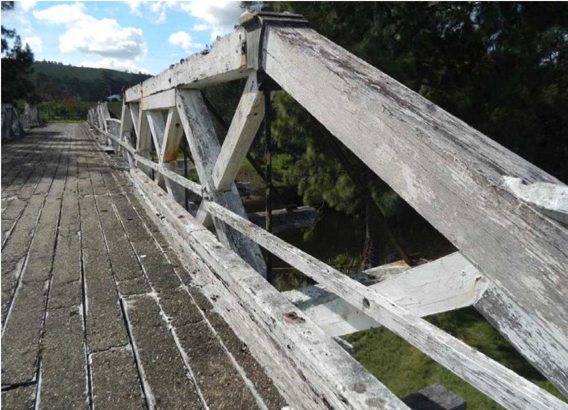
Figure 3-44: Photograph showing broken railings on truss span.
