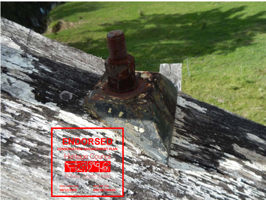
Figure 3-20: Photo of wrought iron bevelled washer and short tension rod.
