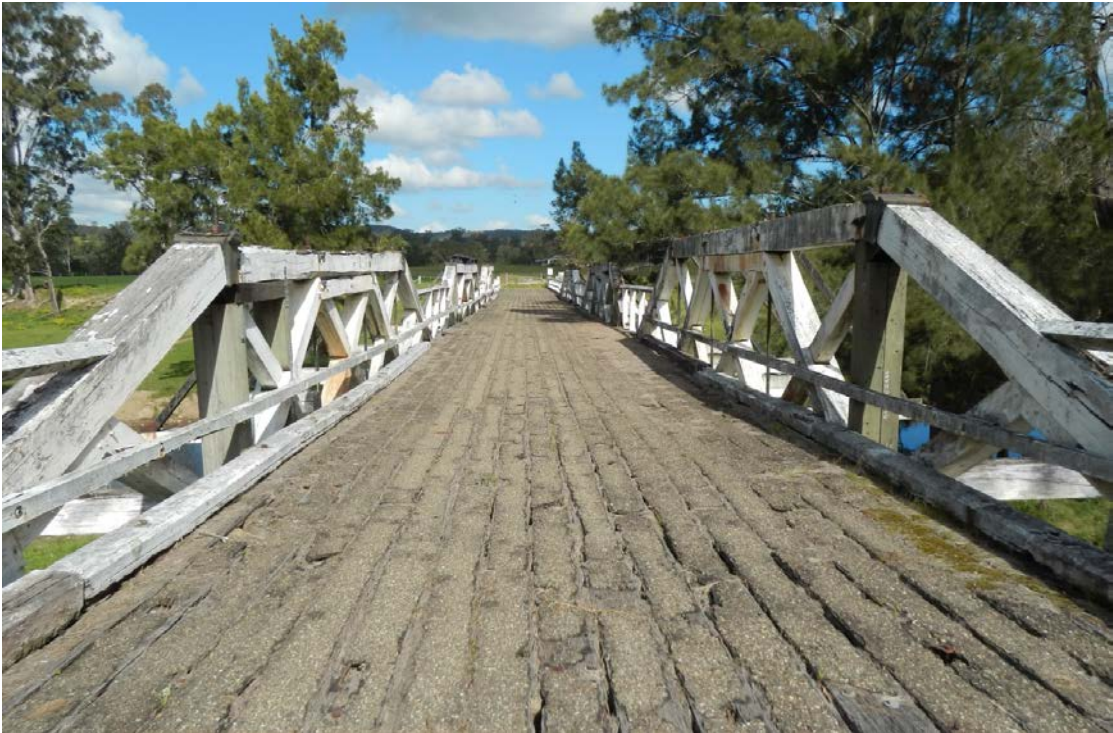
Figure 3-12: Photo of additional timber props and general dilapidation.
