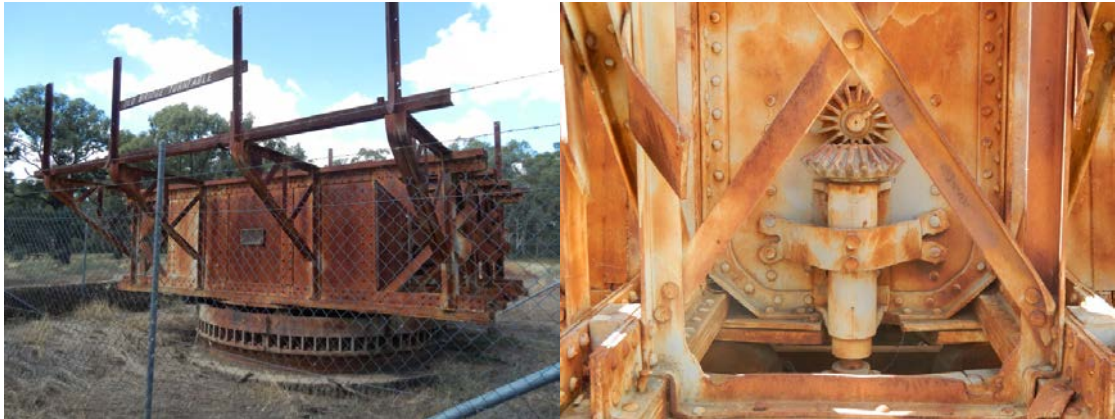
Figure 2-19: Remains of Hay Bridge, Murrumbidgee River today.
