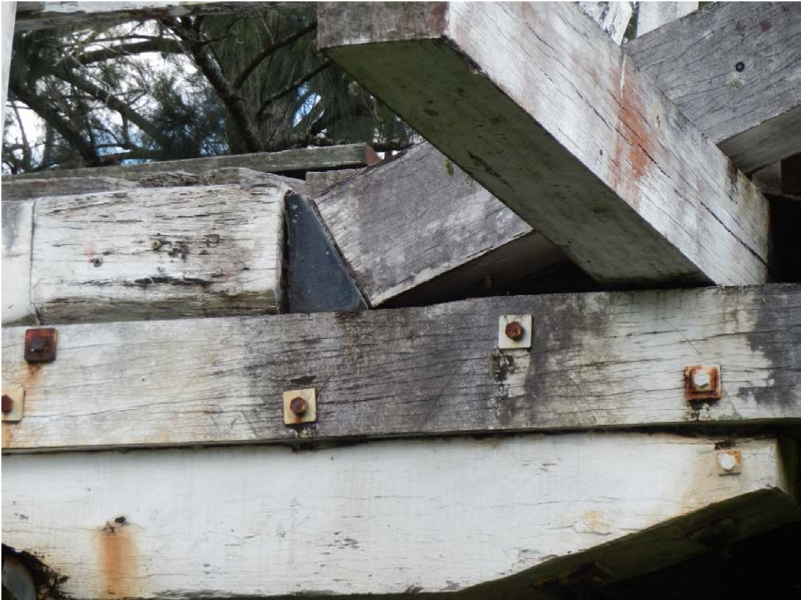
Figure 3-17: Photo of tear drop shaped cast iron shoe largely obscured.
