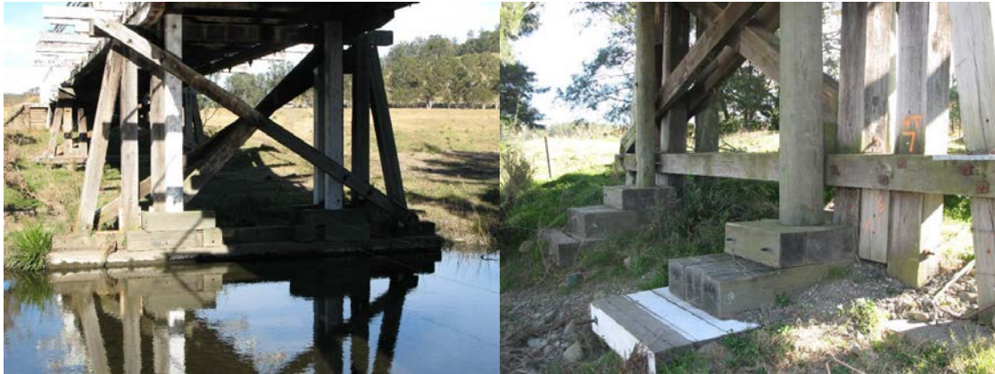
Figure 3-48: Photograph of messy modifications to piers 4 & 5.
