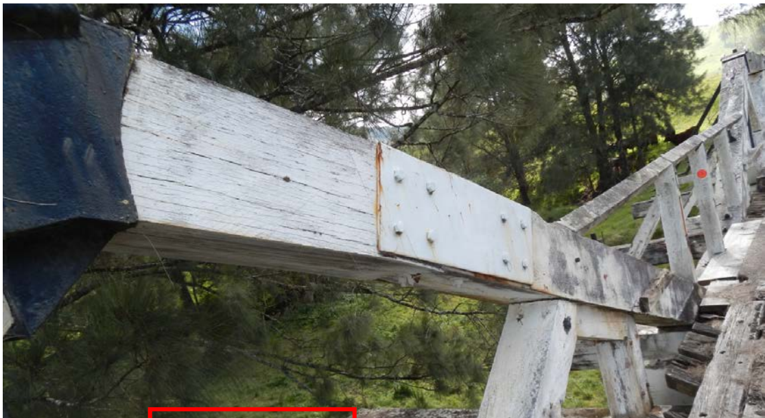
Figure 3-2: Photo of metal side plate and additional bolts on principal.
