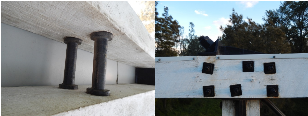
Figure 4.5: Left: Original metal spools; Right: no notching under washer blocks (source: author 2013)
