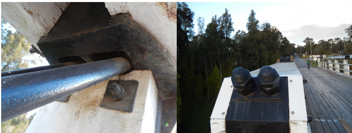
Figure 4.4: Left: Original timber notching at anchor blocks; Right: Introduced flashing (source: author 2013)
