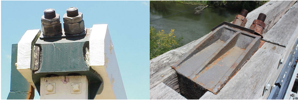
Figure 7.9 Photographs of broken anchor blocks and washer blocks on other de Burgh trusses (source: RMS)
