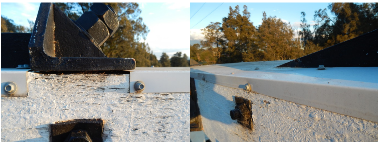
Figure 7.3 Photographs of metal flashing and attachments to top chord timber (source: Author, August 2013)
