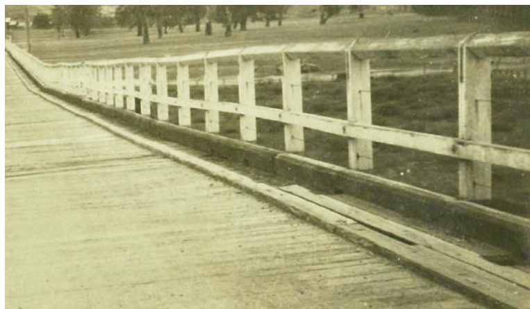
Figure 4.16 Ordnance Fence on Prince Alfred Bridge 1929 (Source: RMS General Bridge File #178.146, vol 1)
