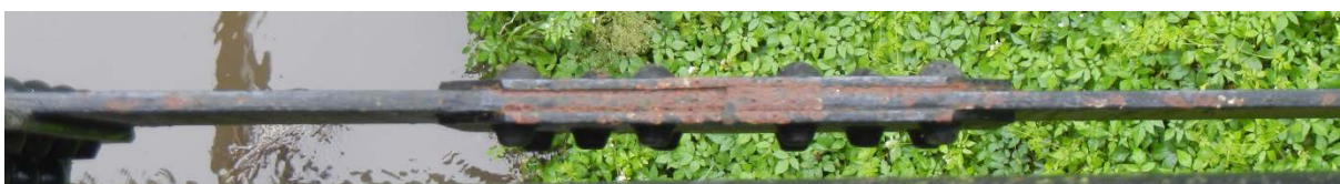
Figure 4.10: View looking down - bottom chord splice connection 1/2" to 3/8" steel plates (source: author 2017)
