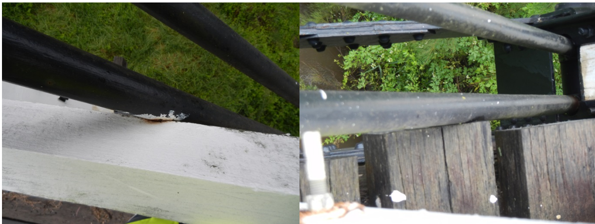
Figure 7.10 Photographs of deterioration of tension rods at Gillies Bridge due to clashes (source: author)
