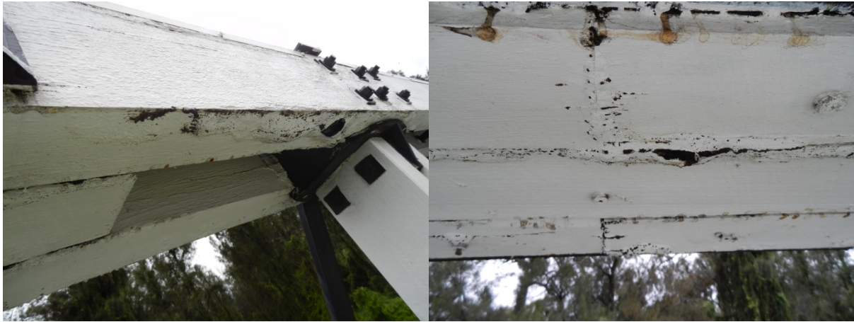
Figure 7.4 Photographs of damage due to non-breathable paint in top chords (source: Author, March 2017)
