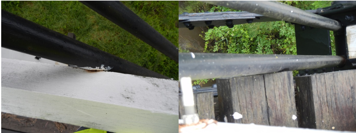
Figure 7.6 Photographs of damage to tension rods from decking and railing (source: Author, March 2017)
