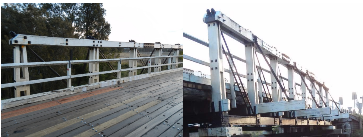
Figure 4.6: Left: Verticals viewed from bridge; Right: verticals viewed from off bridge (source: author 2013)
