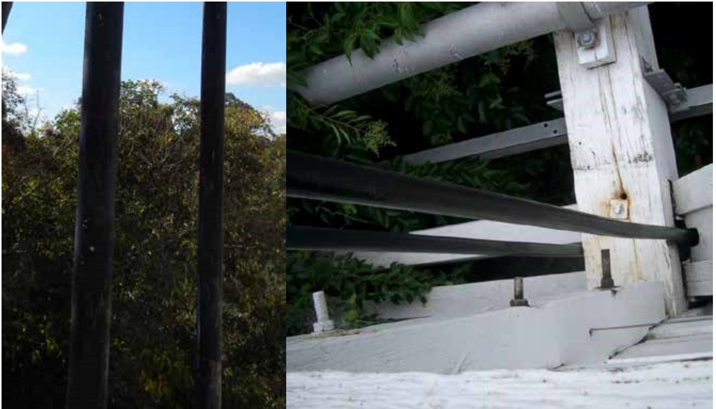
Figure 2-66: Photograph of unequal (left) and damaged (right) tension rods
