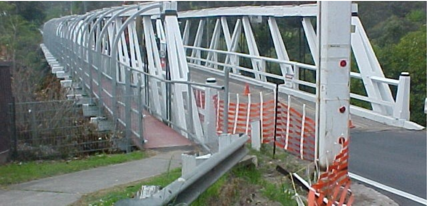
Figure 2-46: Temporary external footway during 2004 repairs
