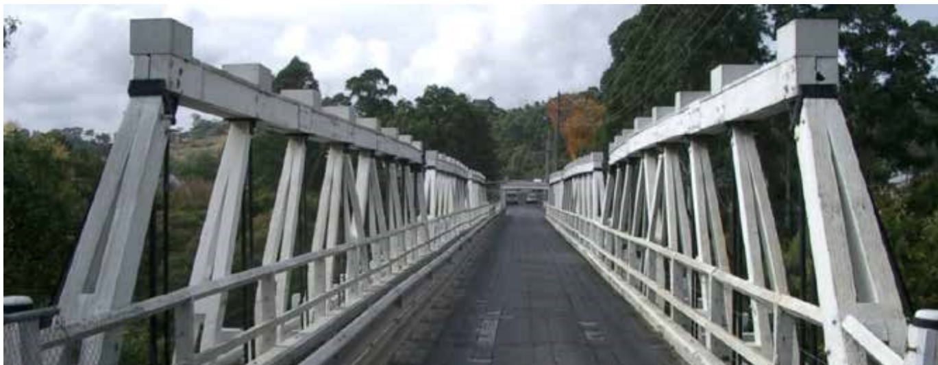
Figure 2-58: Visually dominant “castellated” flashing on top chords
