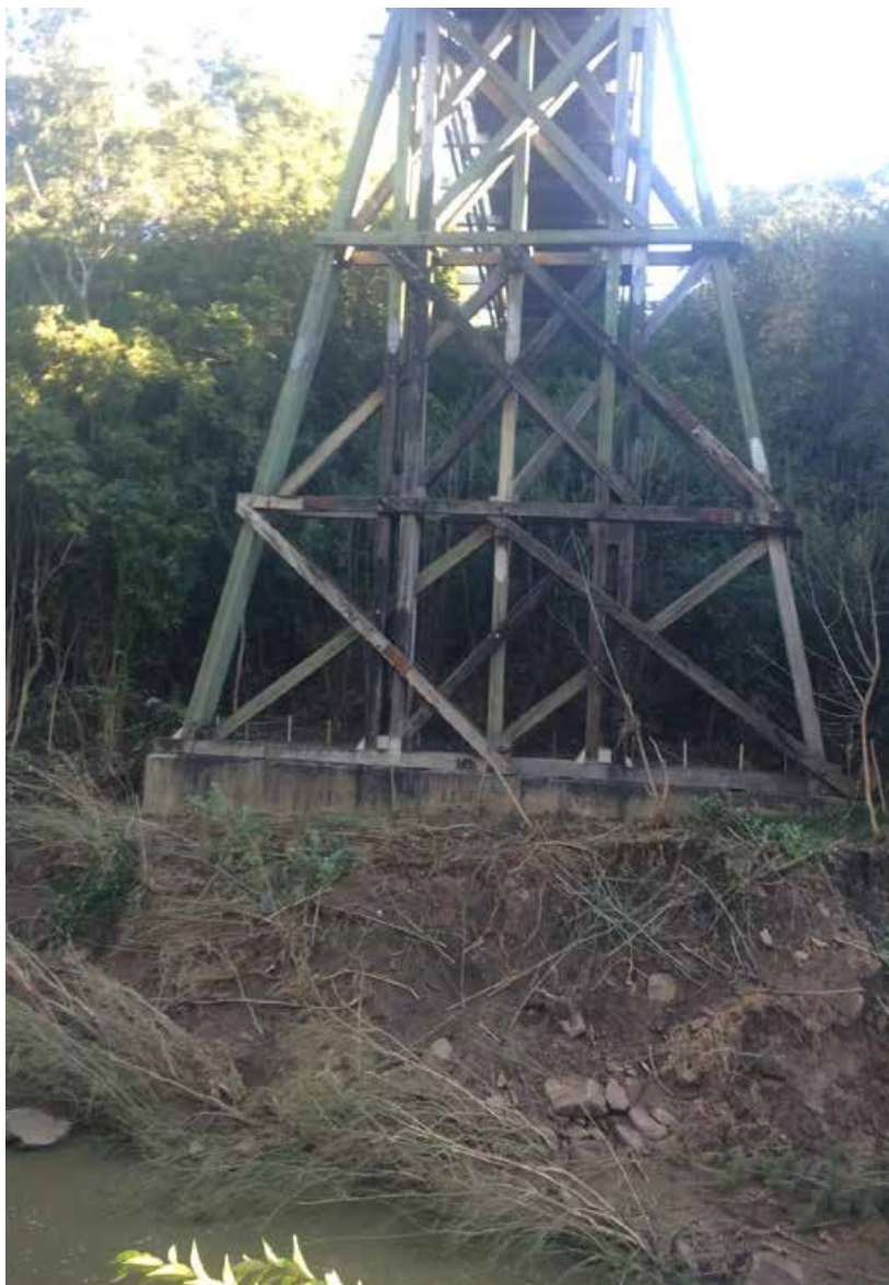
Figure 2-85: Steep embankment due to scour
