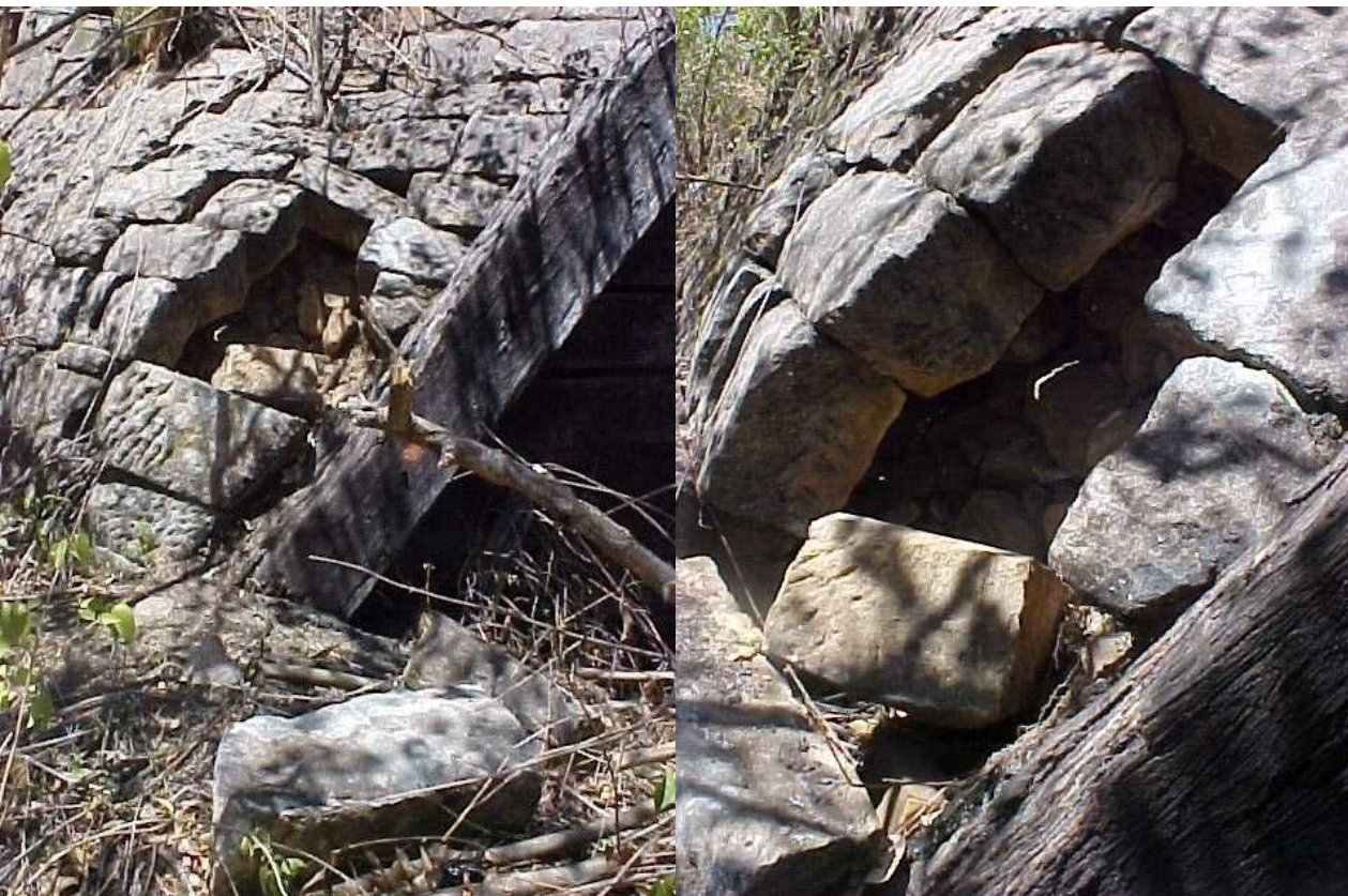
Figure 2-47: Signs of failure of embankment beginning in 2003
