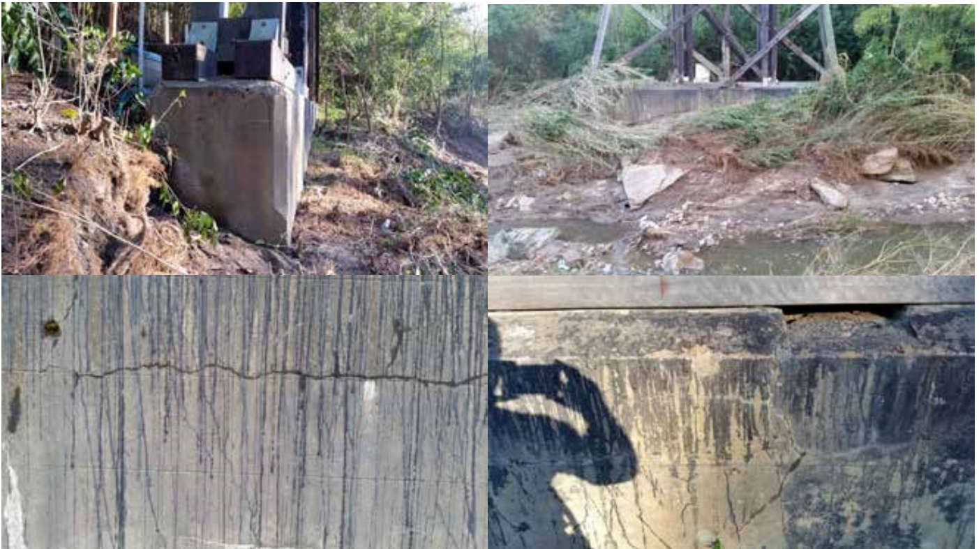
Figure 2-83: Photographs of condition of concrete bases at piers
