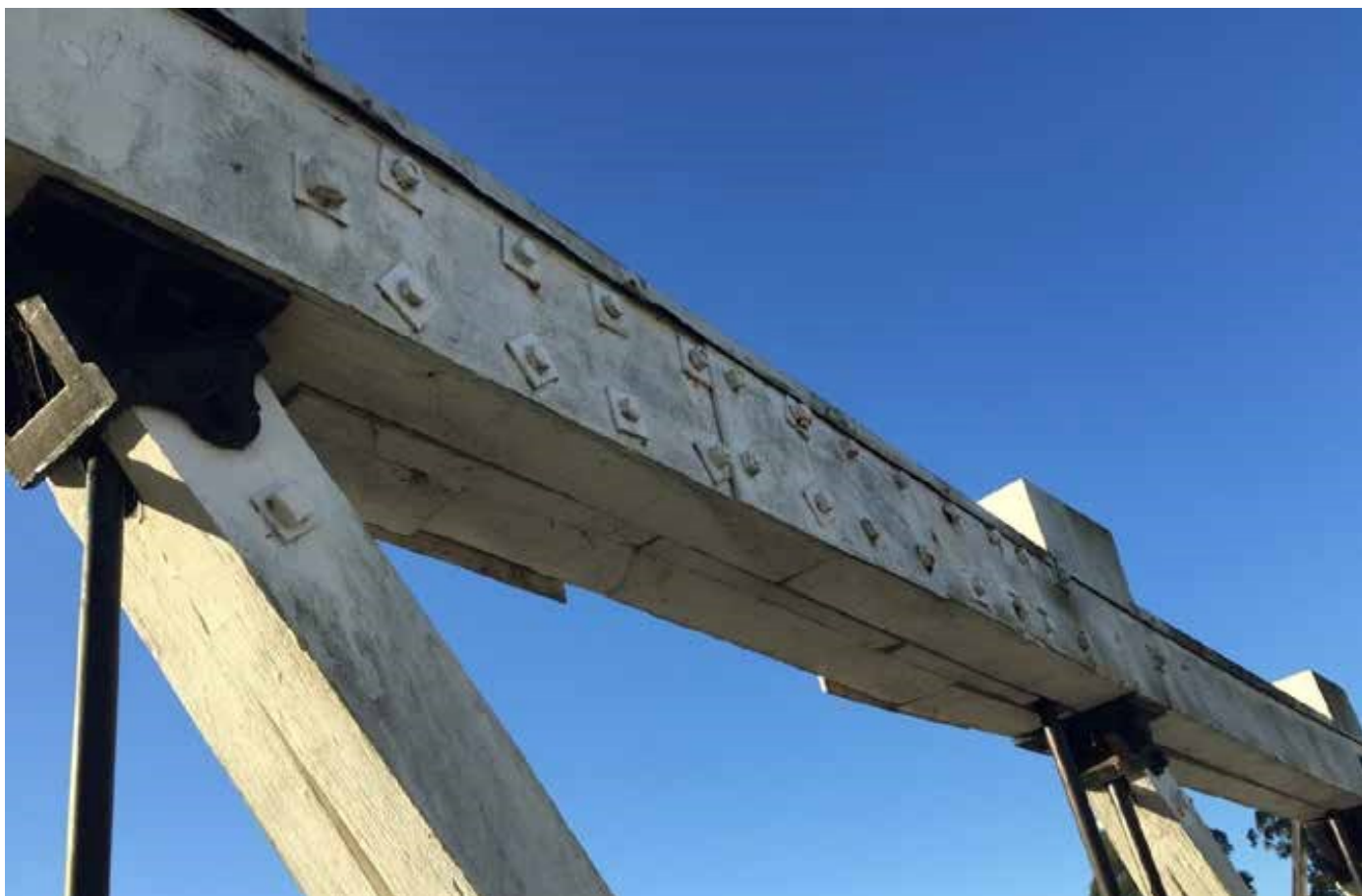
Figure 2-56: Additional splices at G-H in Span 2 Upstream
