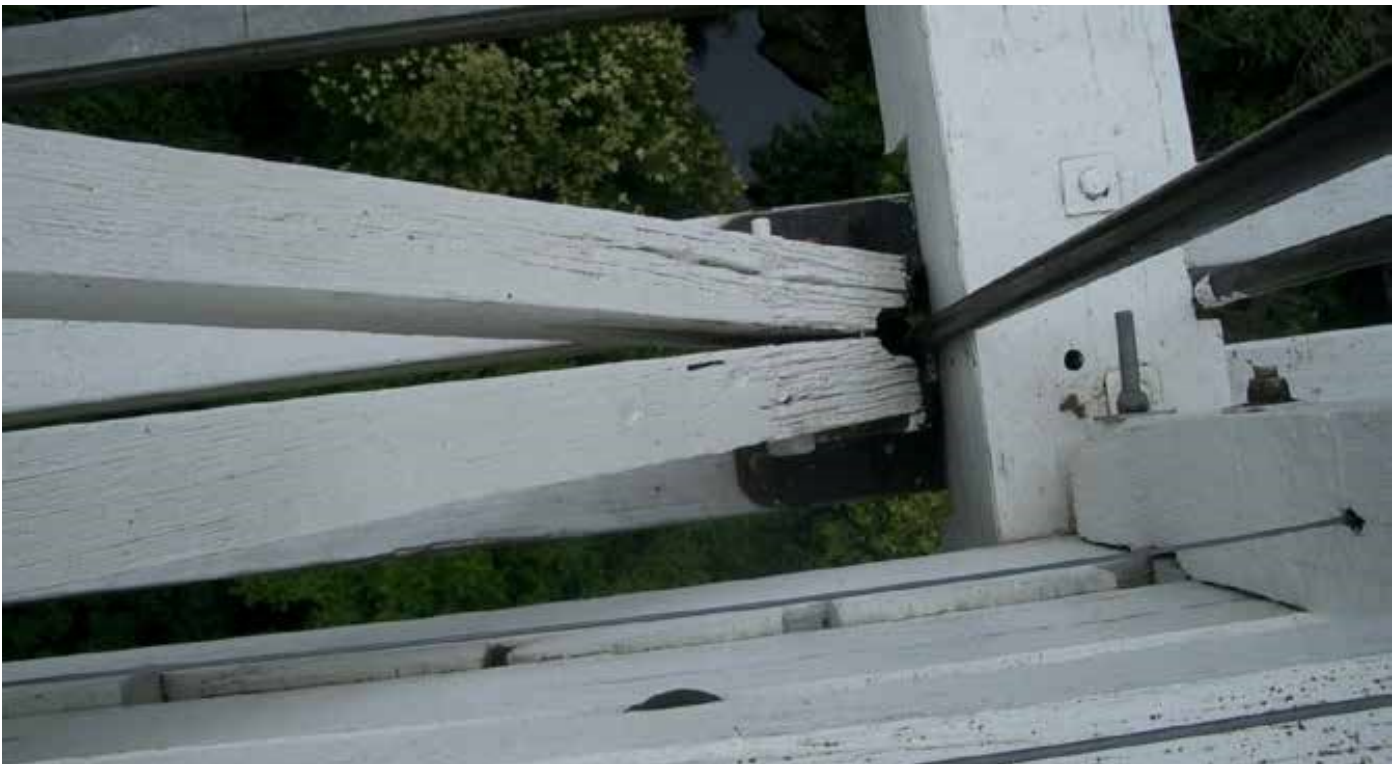
Figure 2-76: Unsightly notching of cross girders at bottom chord locations
