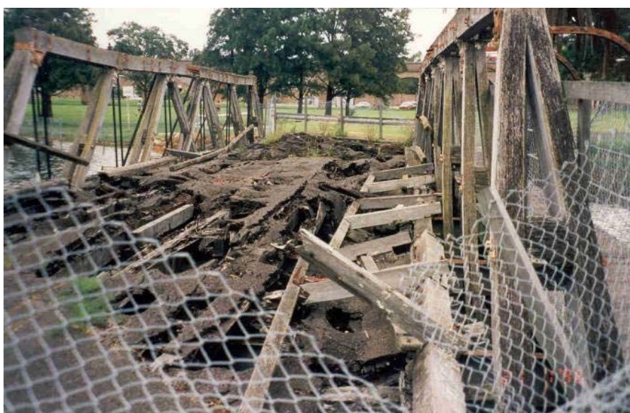
Figure 5.2: Failed pedestrian crossing (source: J. McPhail, 2005)
