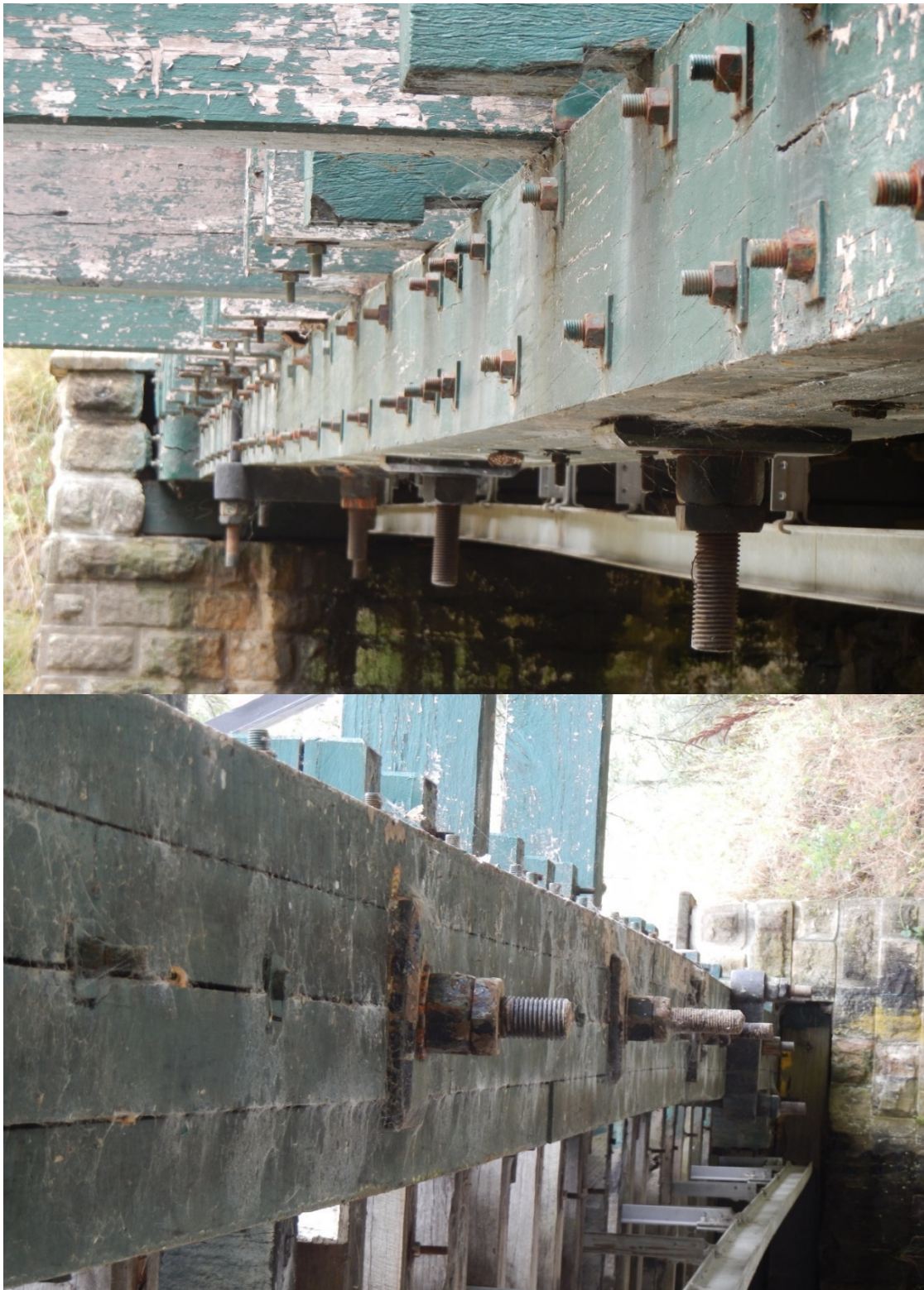
Figure 3-7: Signs of distress in modified laminated timber bottom chords.
