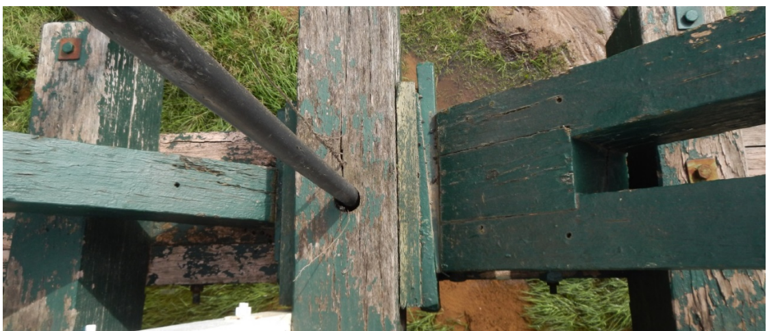
Figure 3-38: Extra timber packing to make up for shrinkage of cross girder.
