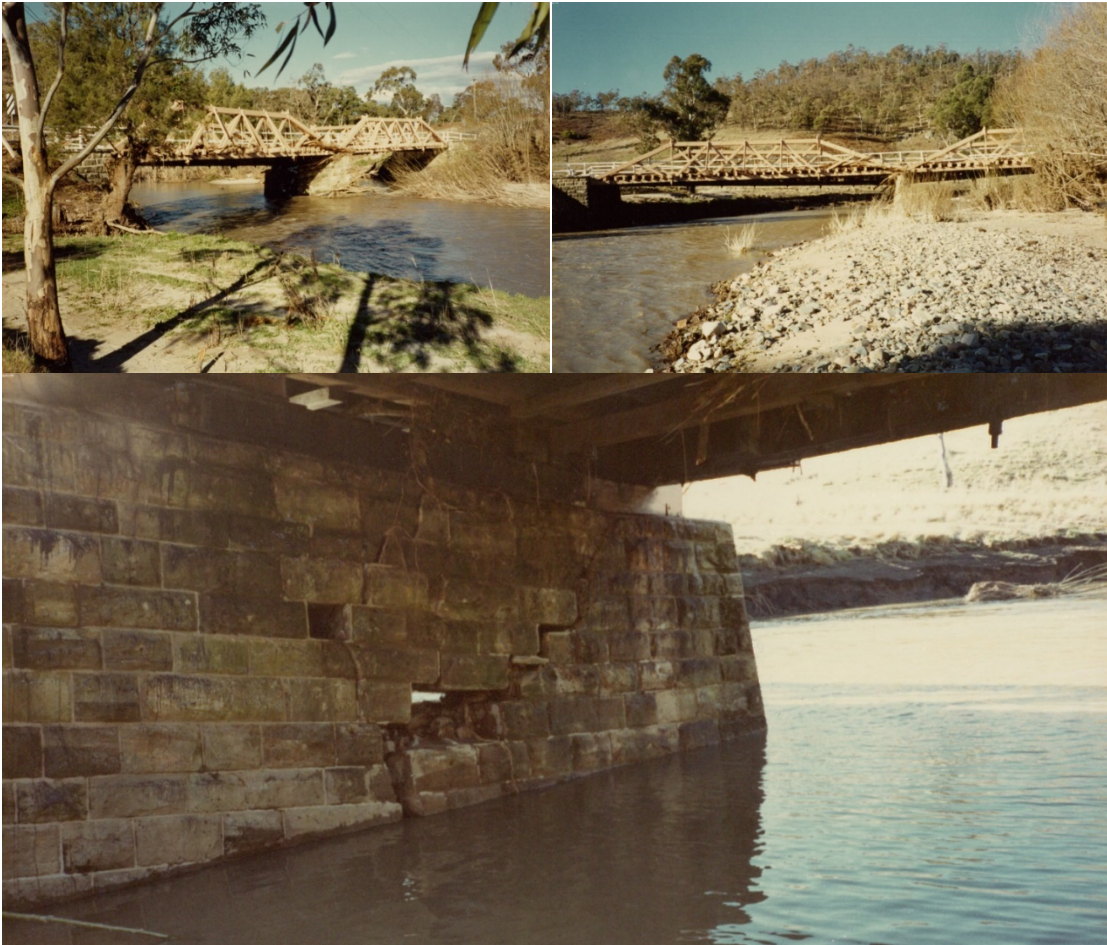
Figure 2-48: Photos of flood damage taken 12 August 1986.
