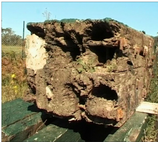
Figure 2-56: Deterioration of timbers removed from McKanes Bridge.
