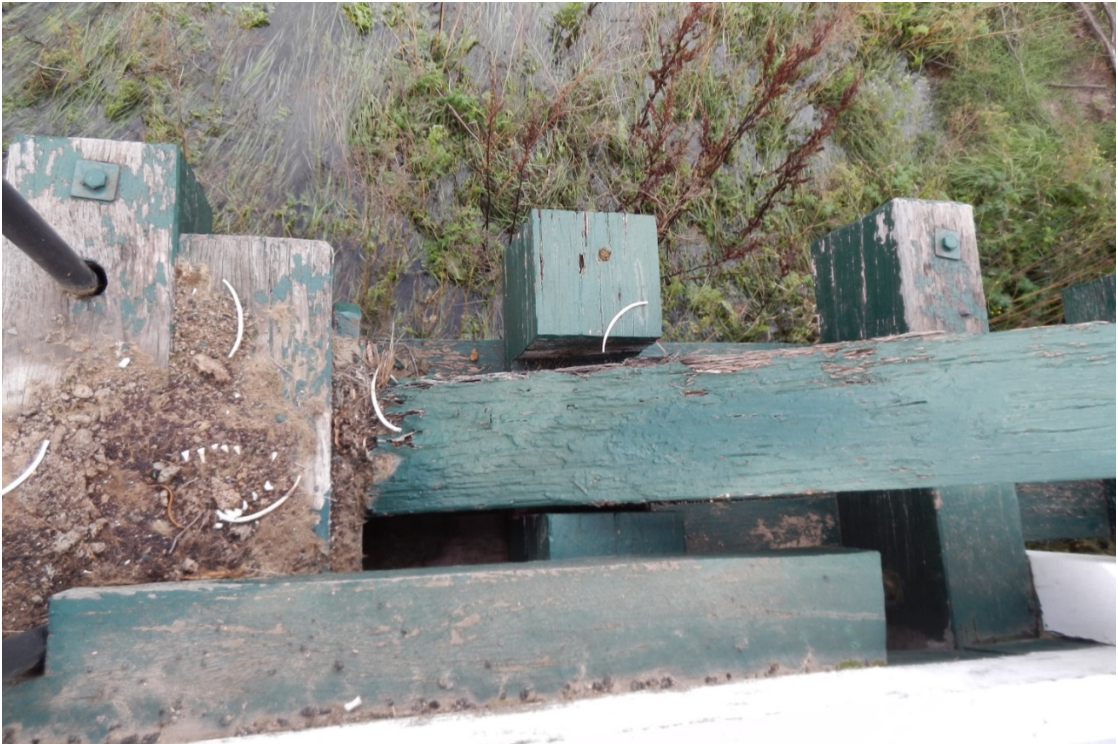
Figure 3-39: Considerable notching of cross girder as per original design.
