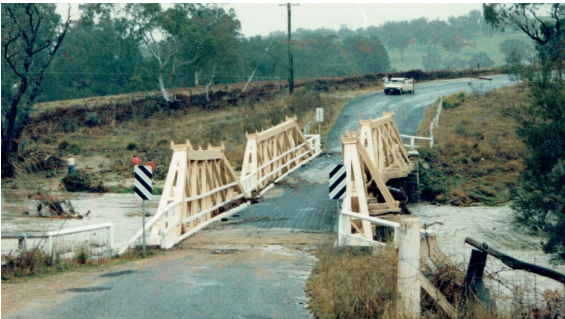
Figure 2-49: Photograph showing flood damage and distortion
