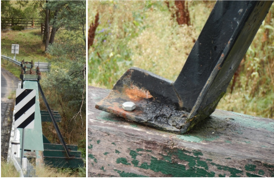
Figure 3-17: Loss of alignment of the trusses due to modifications.
