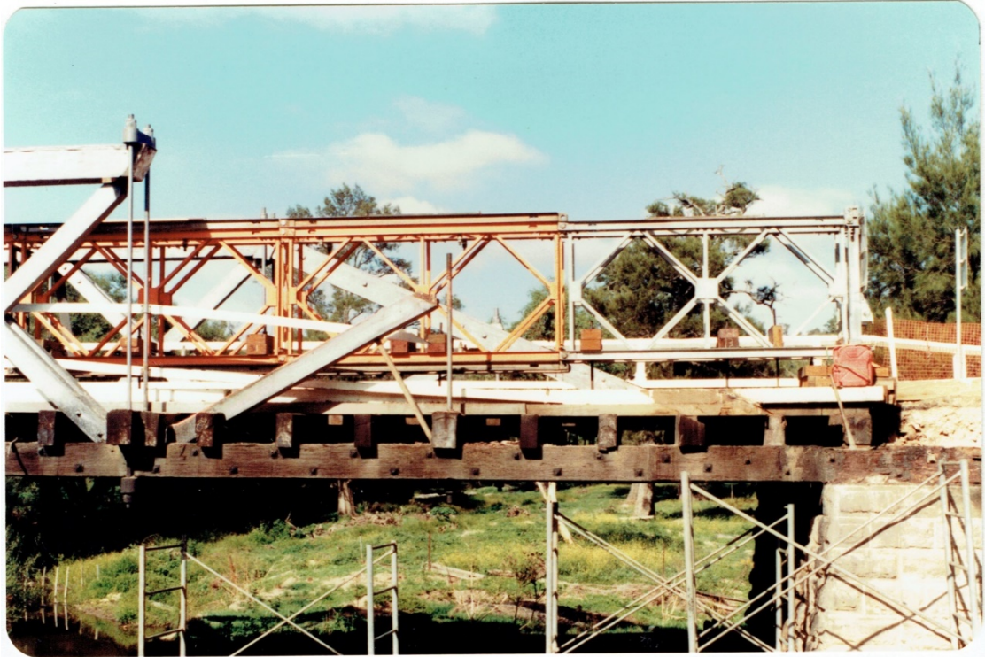
Figure 2-44: Photograph showing replacement of principal in 1982 which required temporary removal of the top levels of stone in the masonry abutment.
