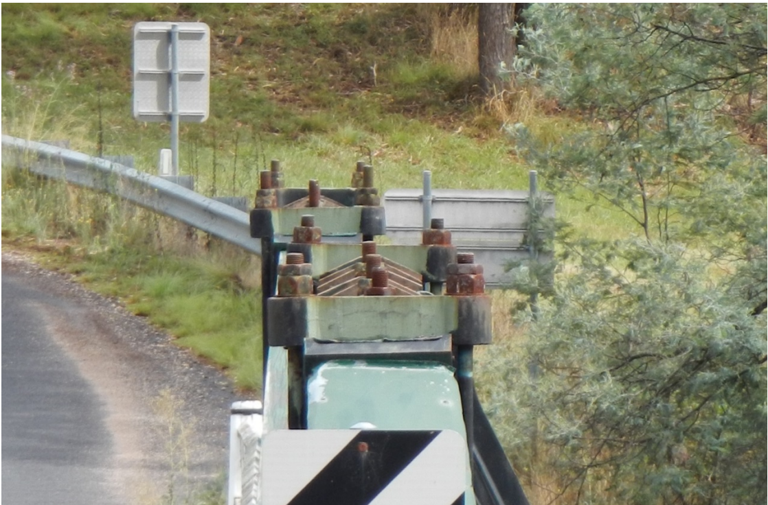
Figure 3-28: Photograph showing corrosion at tops of tension rods and nuts.
