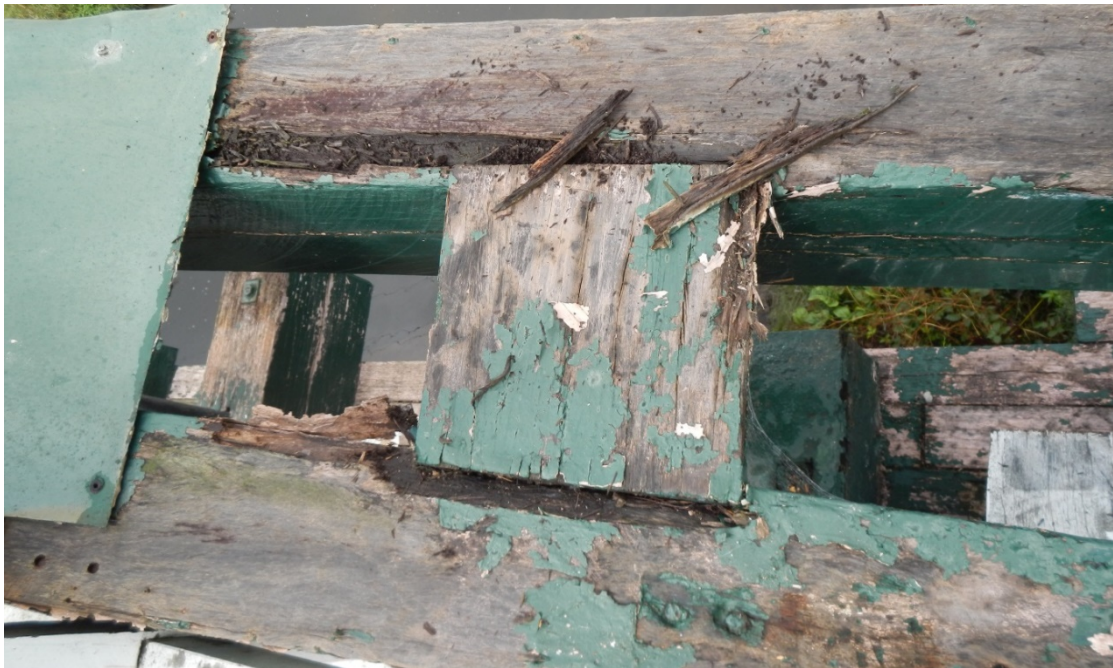
Figure 3-13: Deterioration of flitches of principals at spacer location.
