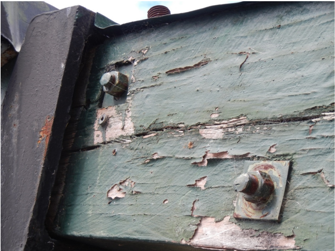
Figure 3-15: Splitting of timber at top of principals and loose fit into shoe.
