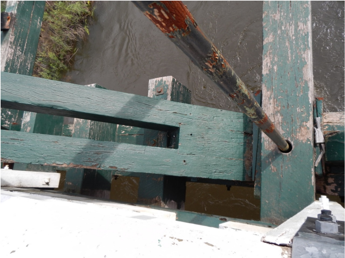
Figure 3-27: Photograph showing paint loss and corrosion of tension rod.
