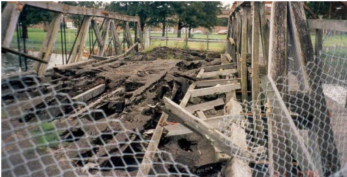
Figure 5-4: Johnston's Creek Bridge, failed pedestrian bridge at Glebe.
