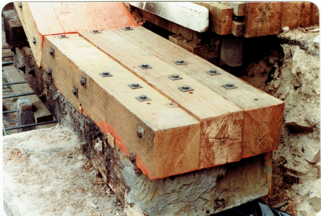
Figure 2-45: Photograph showing new principal and butting blocks being installed and connected to deteriorated laminated timber bottom chords in 1982
