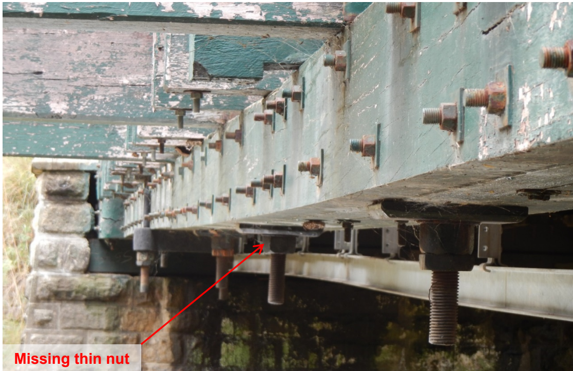
Figure 3-23: Photograph of typical arrangement of nuts with one missing.
