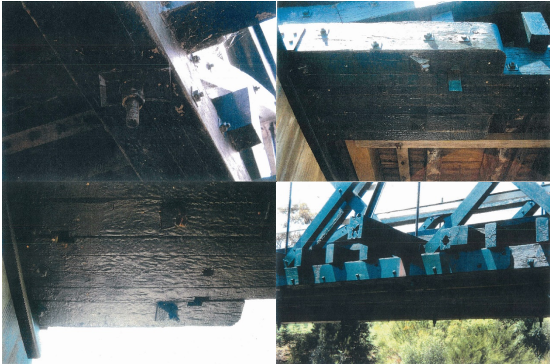
Figure 2-54: Photos of deterioration and damage in 1998.
