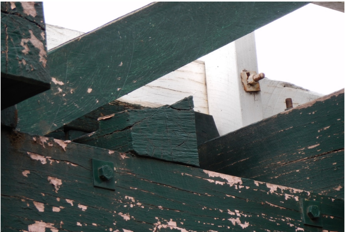
Figure 3-40: Part of secondary cross girder missing due to failure at notch.
