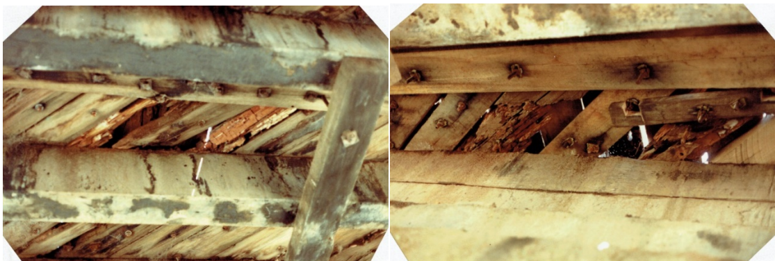
Figure 2-42: Poor condition of diagonal decking in 1981.
