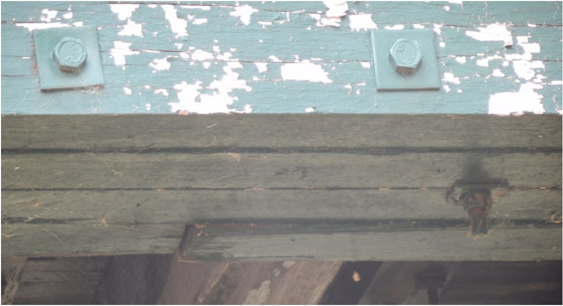
Figure 3-6: Signs of distress in modified laminated timber bottom chords.
