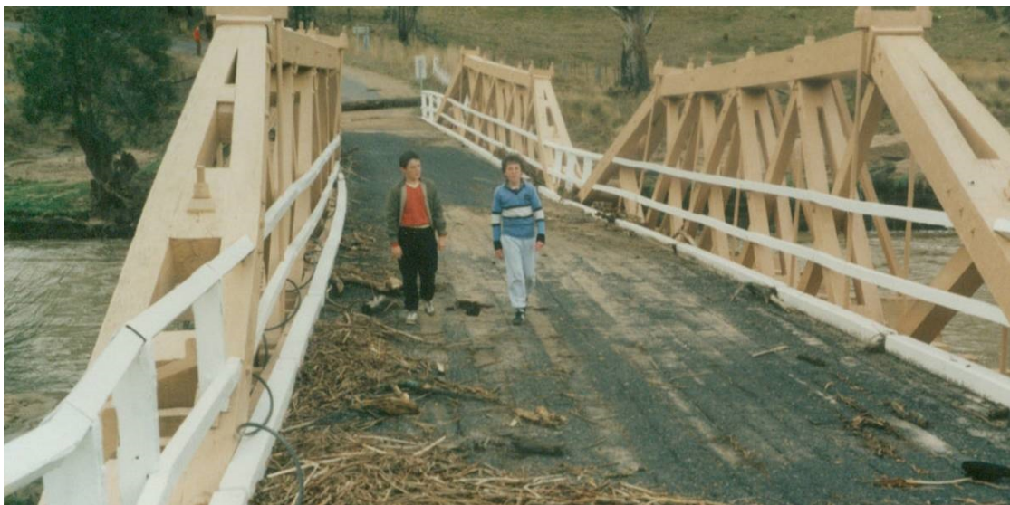
Figure 2-46: Photos of ineffective bridge closure after flood damage.
