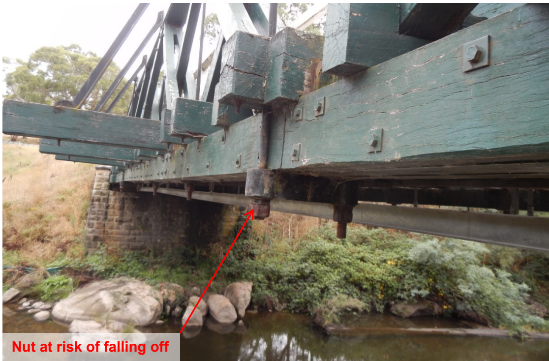
Figure 3-24: Photograph with nut order as designed but close to falling off.
