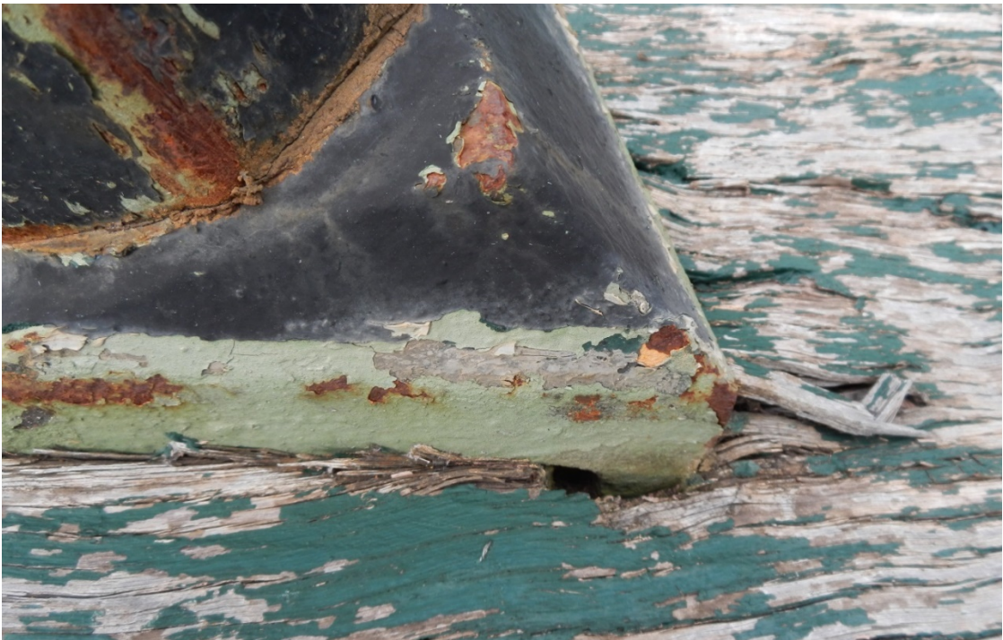
Figure 3-16: Crushing of timber spacer in principal at tension rod location.
