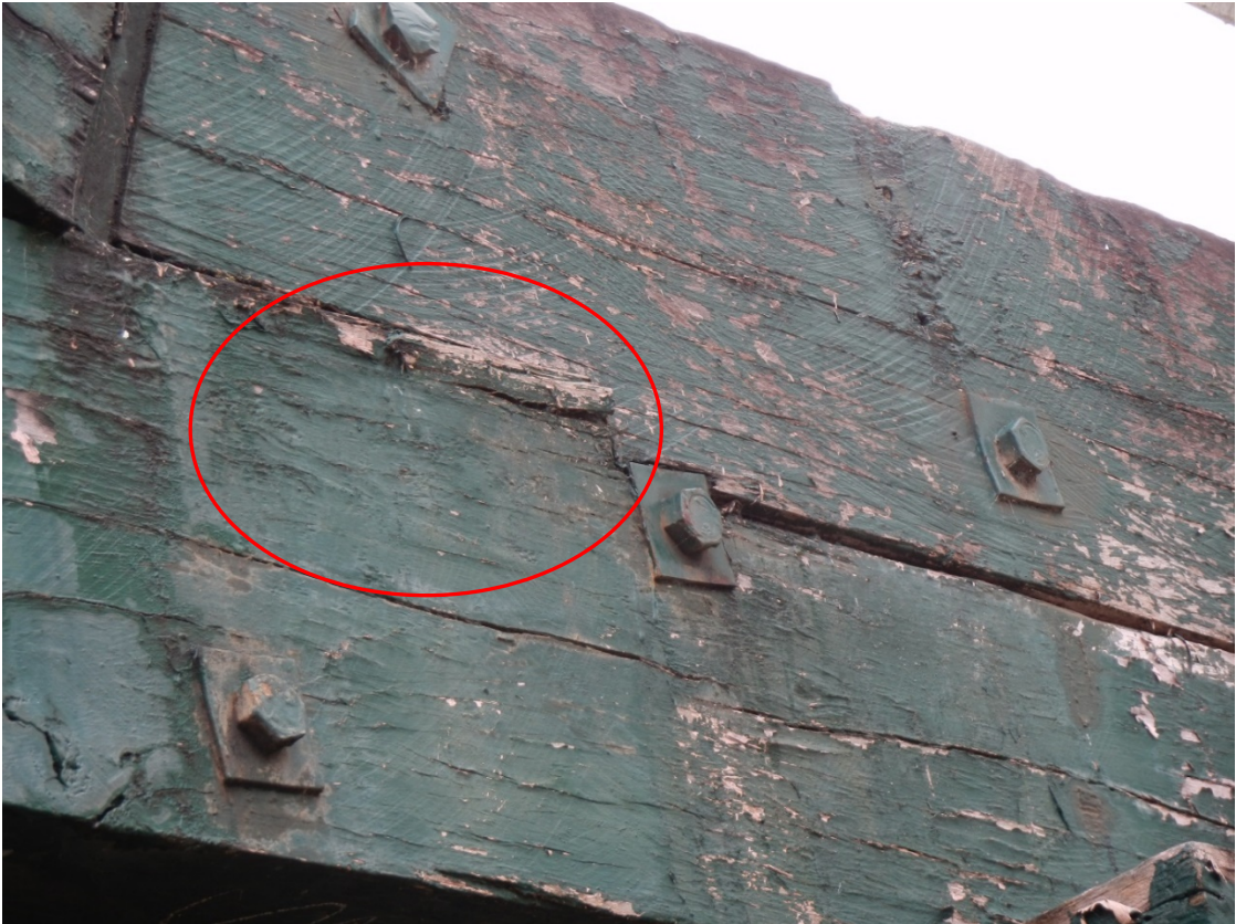
Figure 3-8: Crushing of timber at bottom chord to butting block connection.
