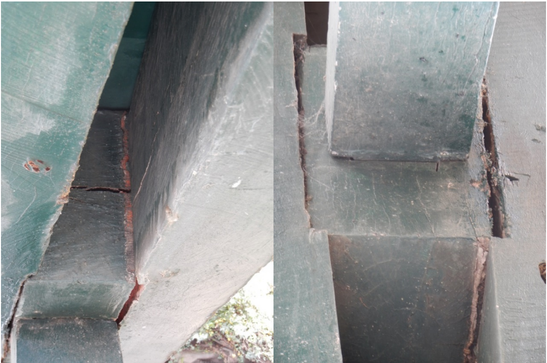
Figure 3-14: Opening of joints and loss of alignment in principals.
