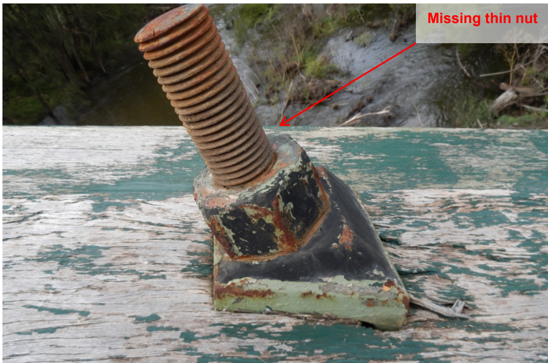
Figure 3-25: Photograph of top of short tension rod with thin nut missing.
